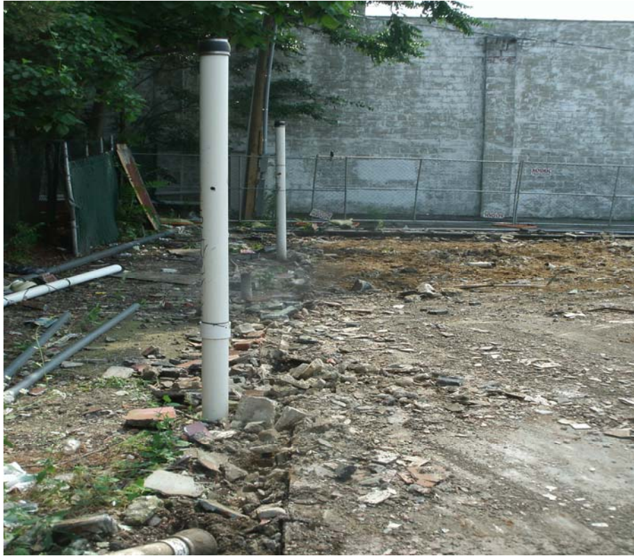
Photo 7 – Sub-slab depressurization piping for former building
