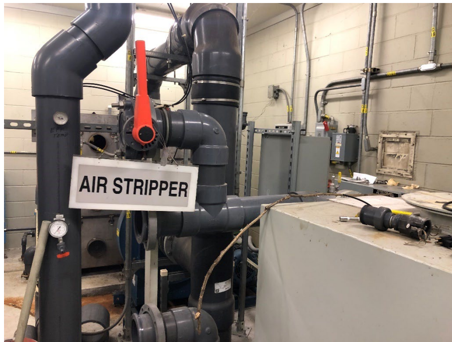
Air stripper process piping, partially decommissioned
