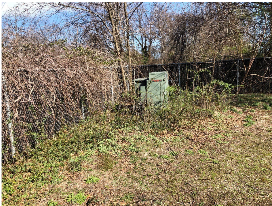
Electrical transformer in the treatment system yard
