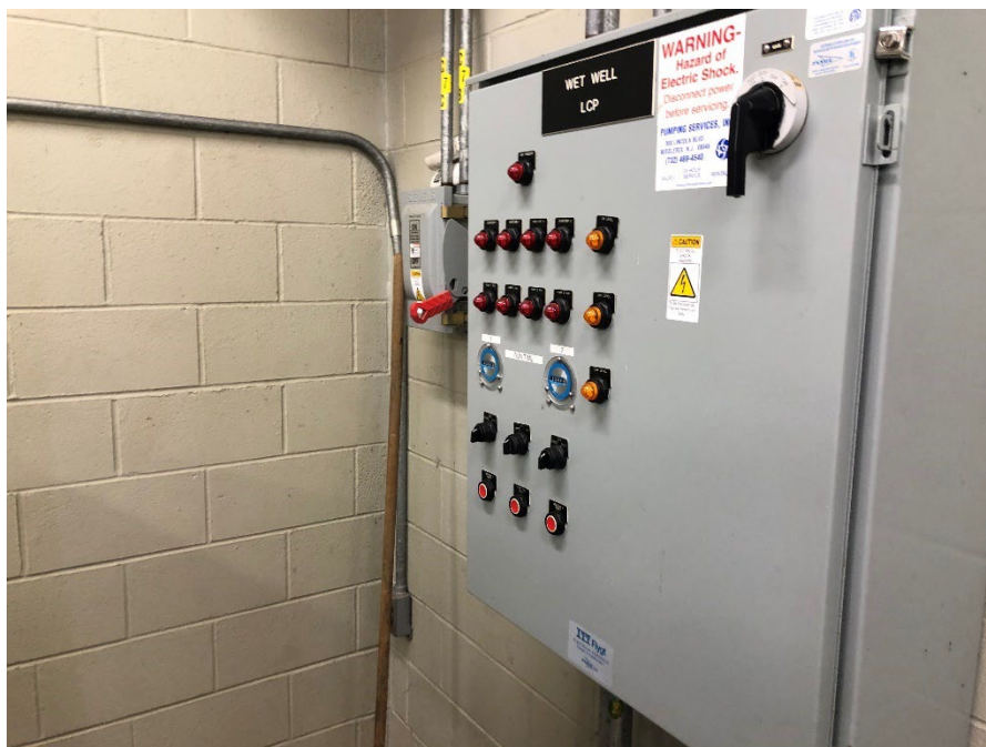
Treatment system electrical panel
