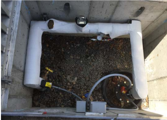
Photograph 3-22: Southern extraction well vault.
