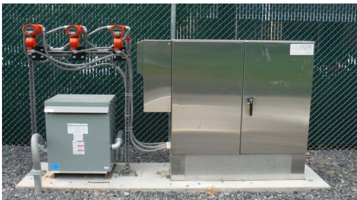
Photograph 3-21: Southern extraction wells transformer and control panel.
