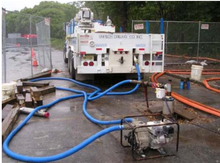
Photograph 3-7: Well disinfection setup.
