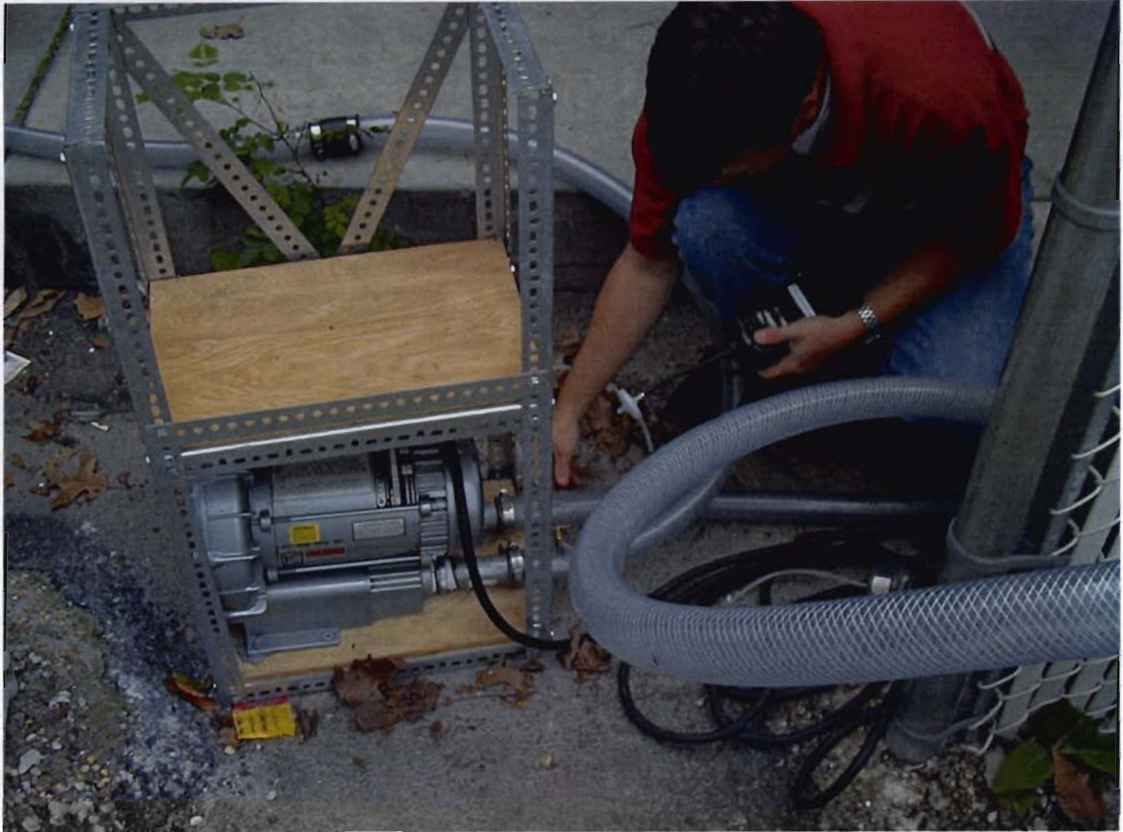
Portable 1 H.P. blower used to test SVE wells at 45 Sea Cliff Avenue site.
