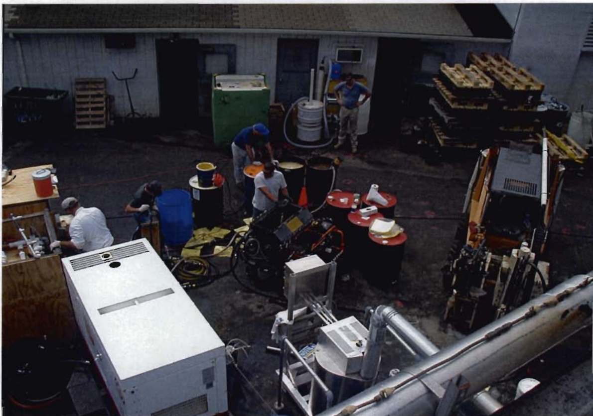
Charging of injection pump with emulsion. Note the stainless steel crossover exhaust between Catalytic Oxidizer and acid scrubber in lower right corner. The corrosion caused by the acidic exhaust stream resulted in the replacement of this section of exhaust with PVC pipe (as discussed in Section 2.1 of this report).
