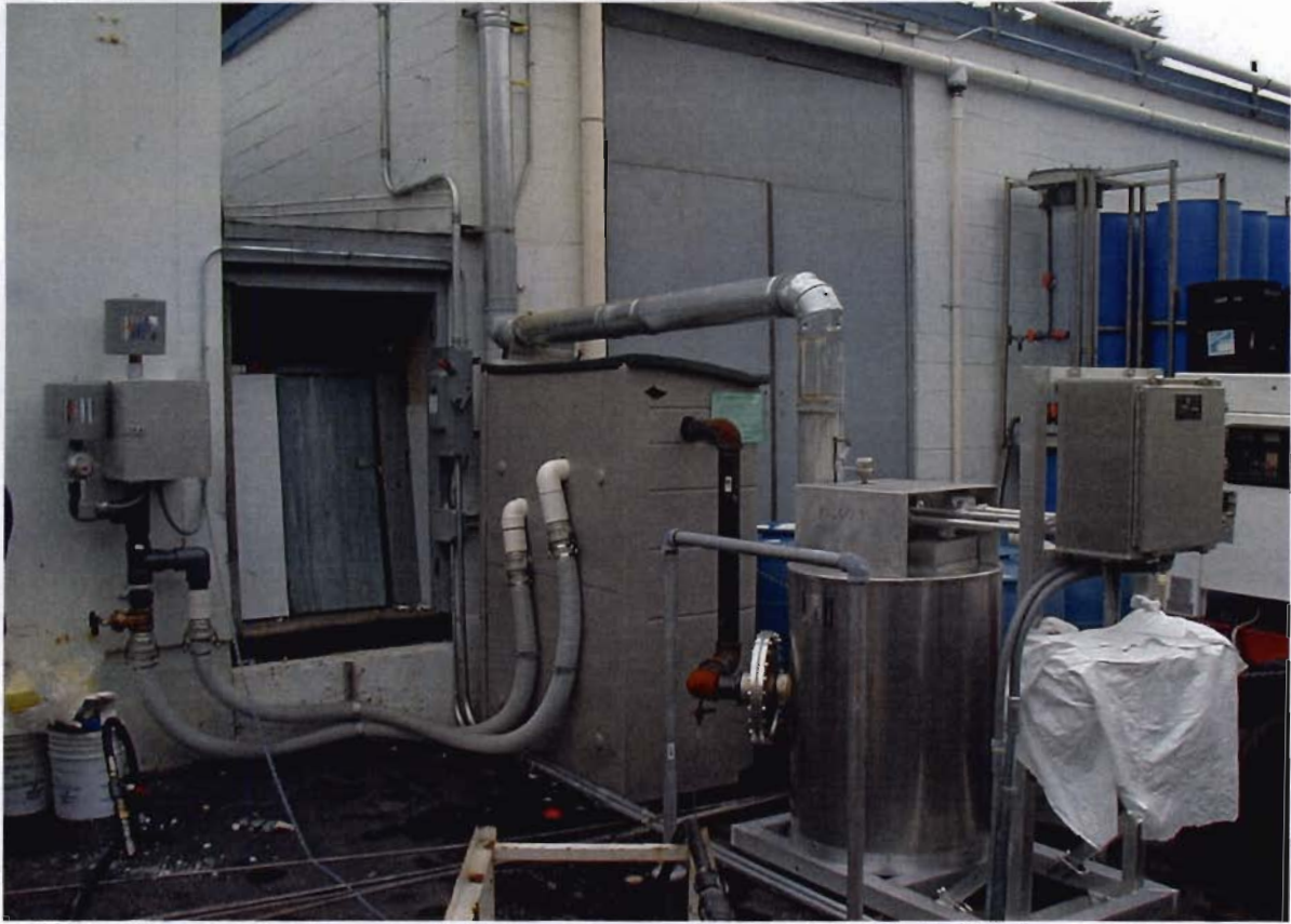
Soil Vapor Extraction System and associated Catalytic Oxidizer installed at 31 Sea Cliff Avenue site.
