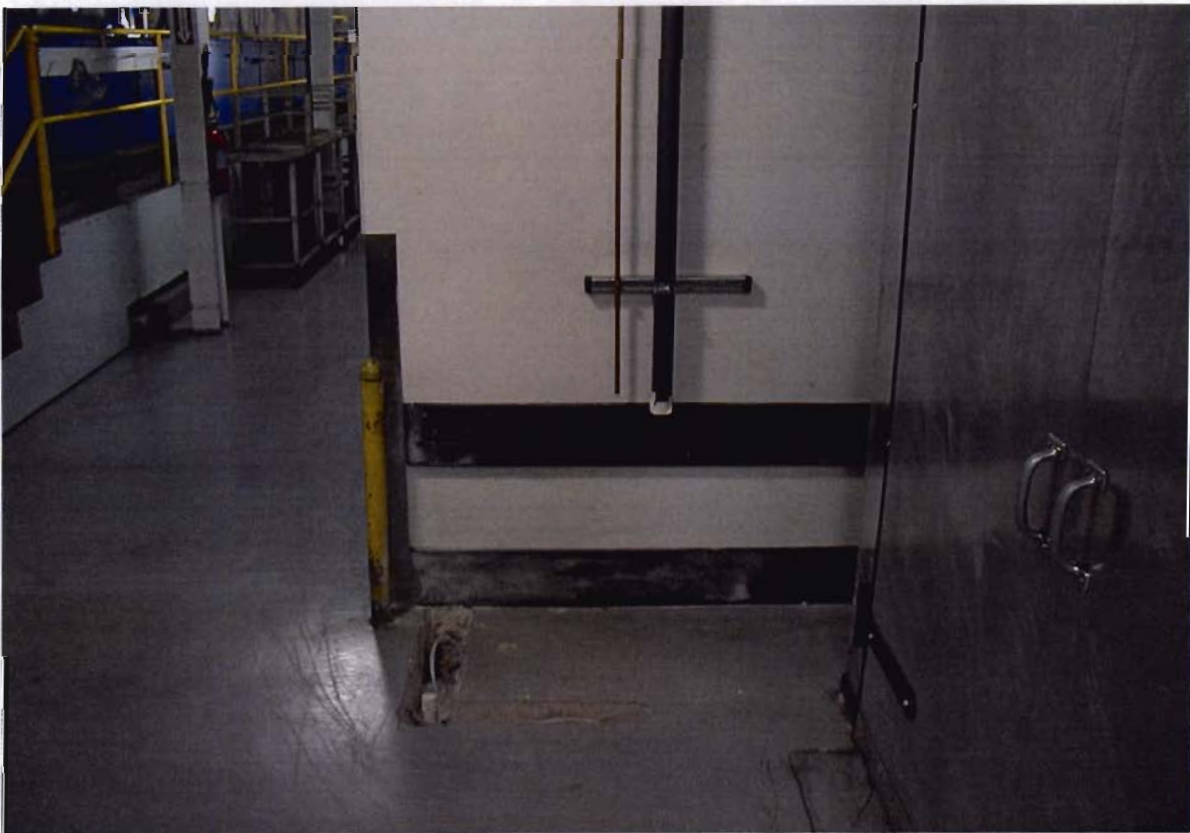
Installation of SVE/AS-4 inside Building 7 at 45 Sea Cliff Avenue site. Note the channel cut that was required through the production floor. The PVC SVE well riser is evident within the channel cut. The polyethylene tubing inside the channel cut connects to the air sparge point. A vehicle-mounted Geoprobe unit (Mule) had to be pushed by hand through the narrow aisle to access this location.
