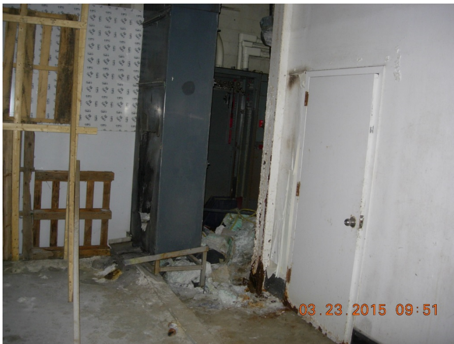
Building 7. Unknown substance on floor
