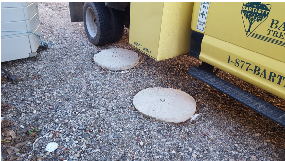
Photograph #10 – Protective concrete discs covering well vaults for monitoring wells MW-2D (left) and MW-2S (right).
