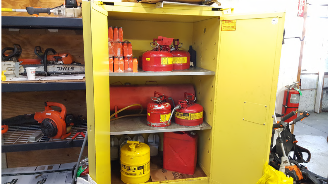
Photograph #7 - Ground floor interior of office/garage building. Flammable storage locker for lubricants, 2-cycle gasoline mix, diesel fuel.
