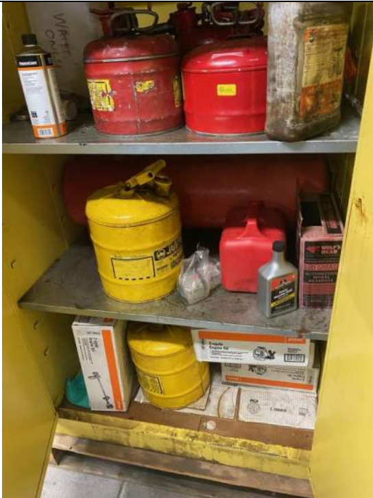
Photograph #8 – Ground floor interior of office/garage building. Flammable storage locker for lubricants, 2-cycle gasoline mix, diesel fuel.
