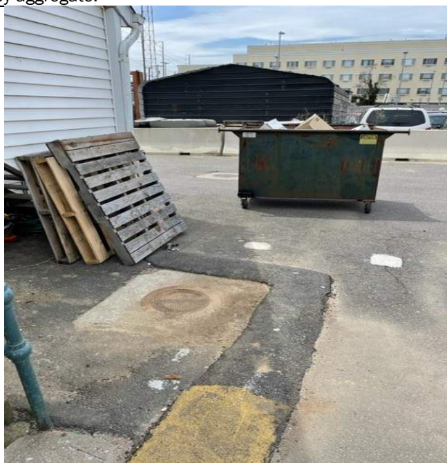
Photograph #3 – Area of remaining subsurface soil contamination, vicinity of former test pit TP-2, under wheeled trash receptacle. Area is covered by asphalt paving.
