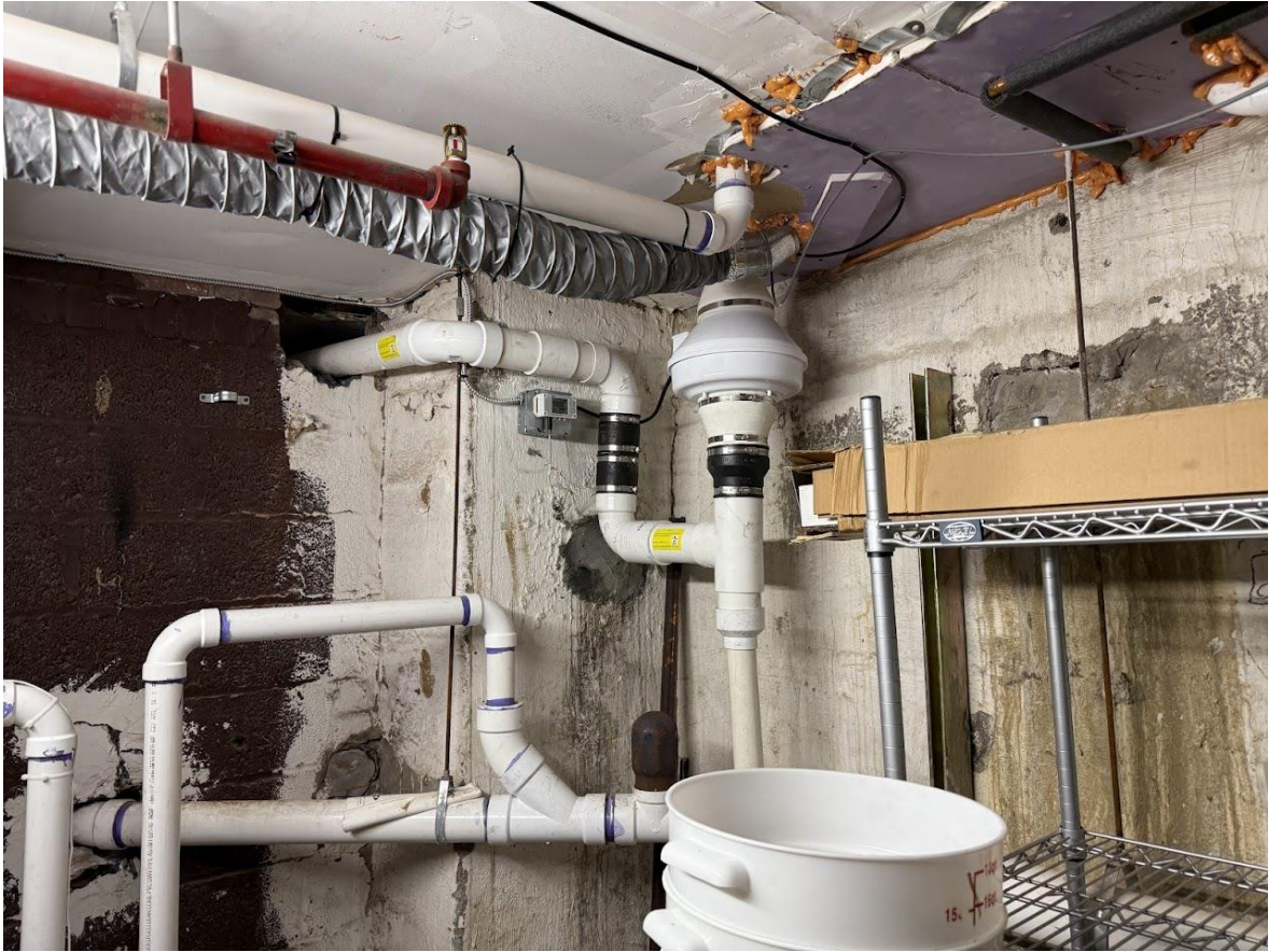
Photo 5, SSDS Fan, Labeling Amp Meter, and Vapor extraction point in basement of Restaurant
