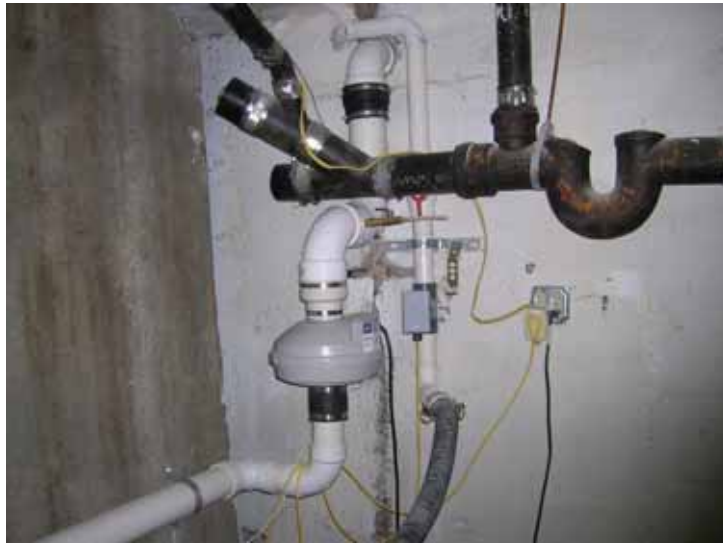
Photo 1 Sub-slab depressurization System Fan and Exhaust (3" and 4" PVC lines) Soil Vapor Extraction System Exhaust (2" PVC line).
