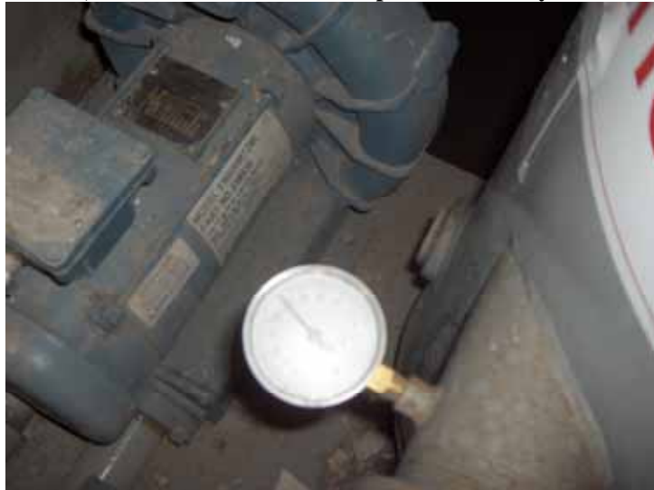
Photo 3, Soil vapor extraction system blower and gauge
