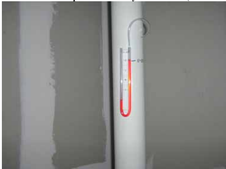
Photo 2, Manometer for sub-slab depressurization system in basement storeroom
