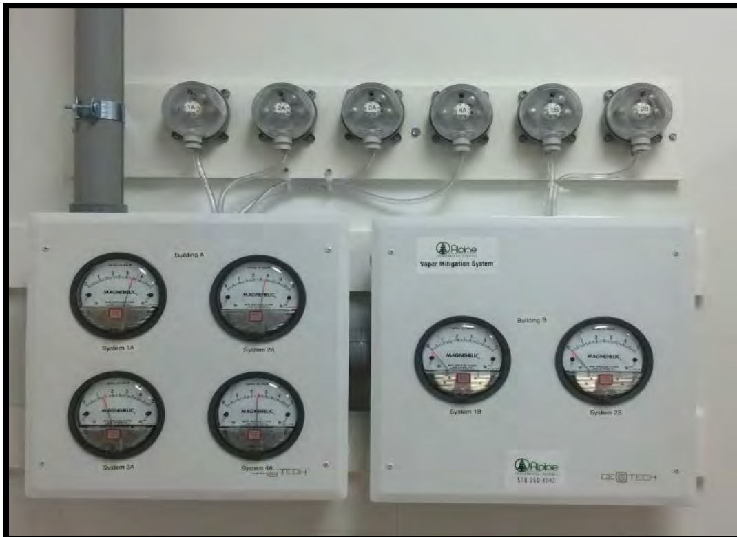
Figure 4.4; Monitoring Panel in the electrical room of the Learn & Play Day Care Center. See Figure V-101 in Appendix A for location. Adjustable pressure switches are located on the top row and mechanical pressure gauges for each sub system in the bottom panels.
