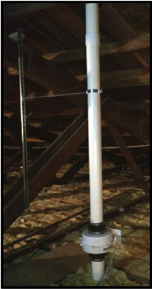
System 2A fan and exhaust piping
