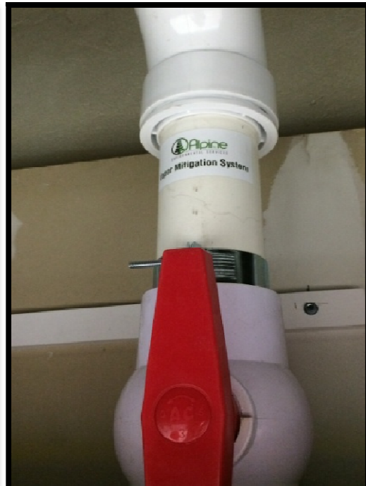
Extraction pipe 2B-1 balancing valve and labeling
