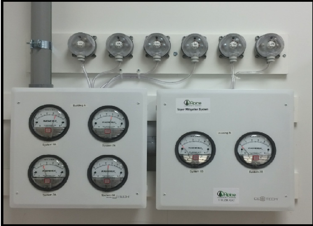
Systems monitoring panel
