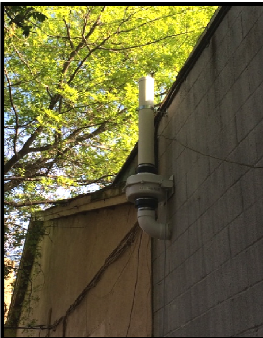
System 2B fan and exhaust piping
