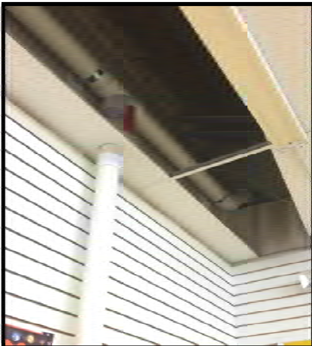
System 1B horizontal piping run
