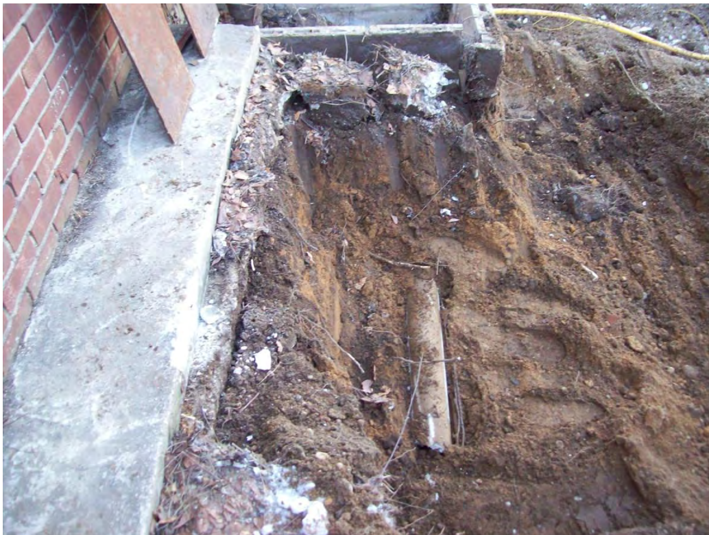
Photo 12. Broken sewer line in excavation.
