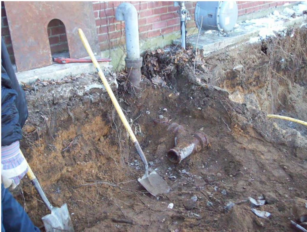
Photo 13. Broken sewer line in western excavation.
