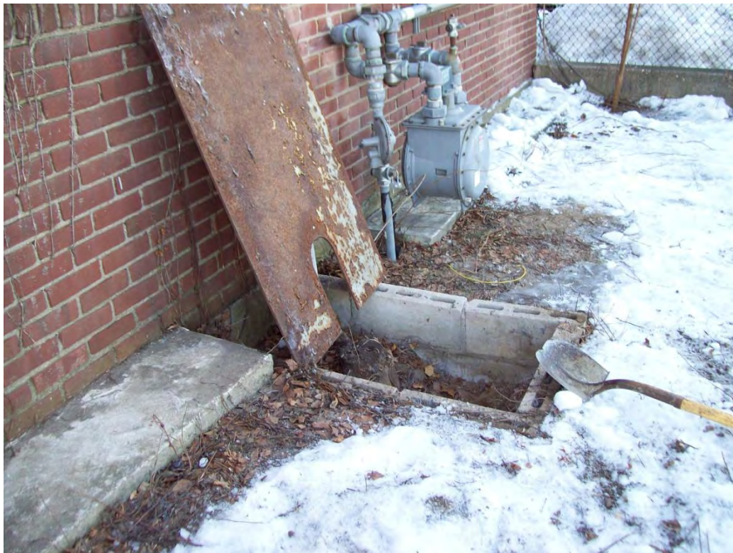
Photo 4. Utility connections on north side of building.
