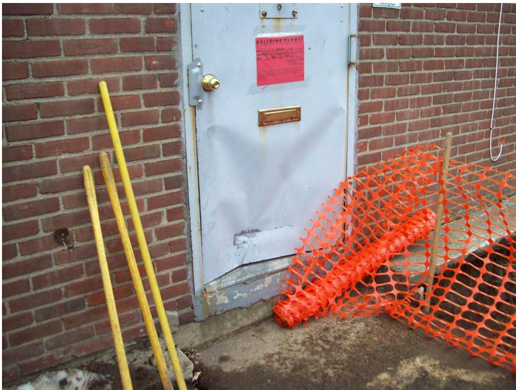
Photo 20. Door damaged by out-rigger of excavator.
