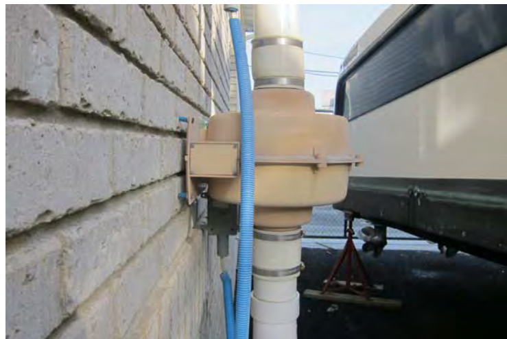
Fan slightly pulling away from building wall
