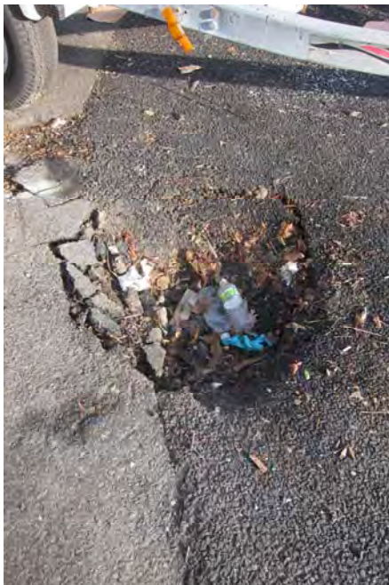
Porous pavement blowout west of warehouse
