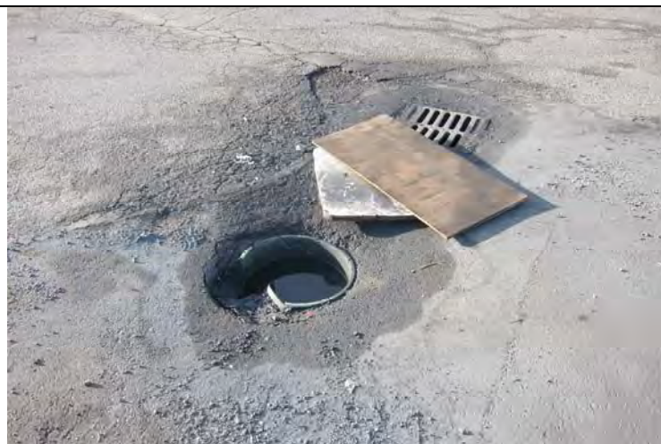
Hole/pipe observed in southeast portion of site
