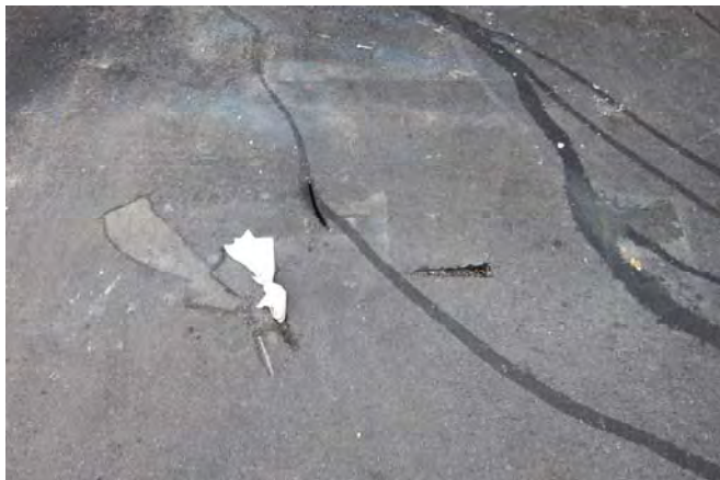
Punctures observed in porous pavement in southeast corner of site- likely from marina operations
