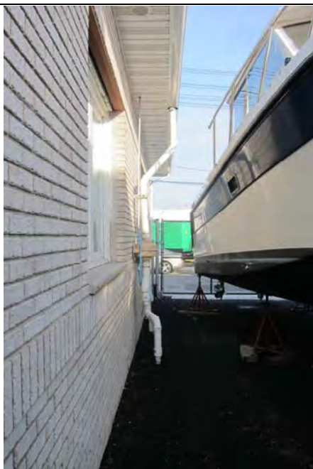
System on east side of office building
