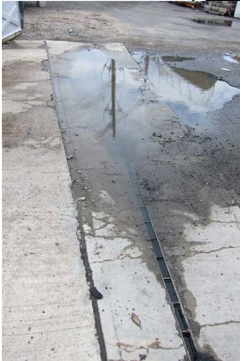
Eastern storm drain clogged from recent storm event
