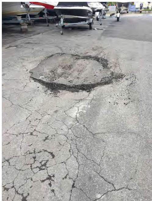
Cracked pavement at site.
