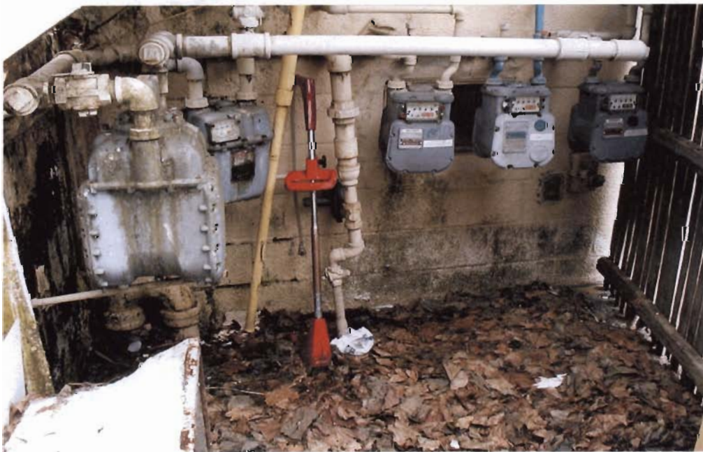
Figure 6 – Rear of 22-26 Railroad Avenue, location of natural gas lines and service meters.
