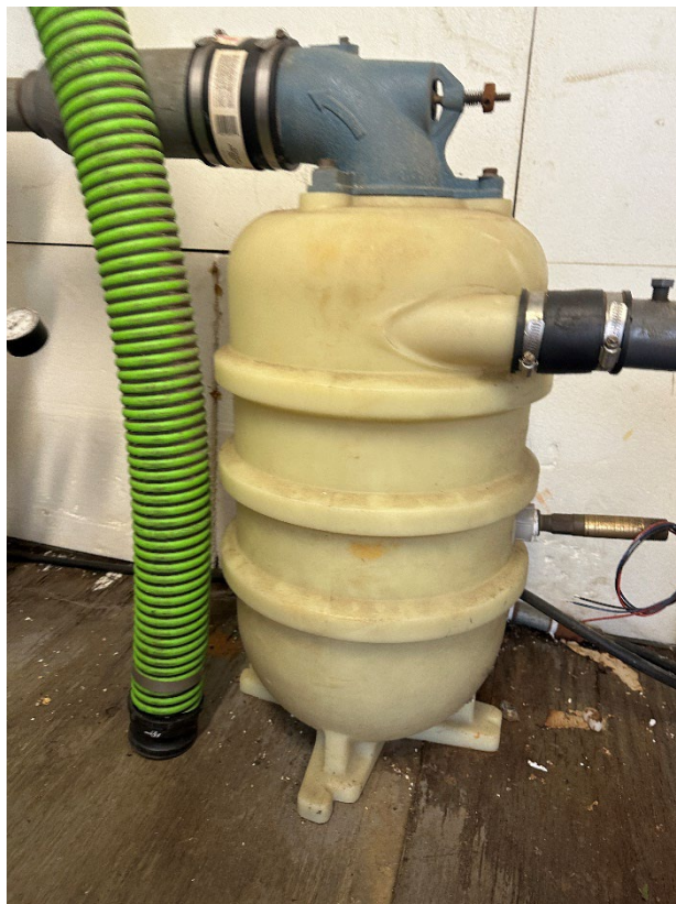
Photograph 2: View of the knockout tank.
