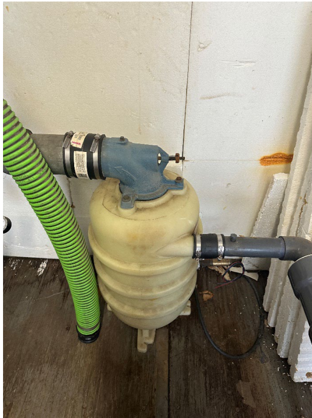
Photograph 3: View of the knockout tank.
