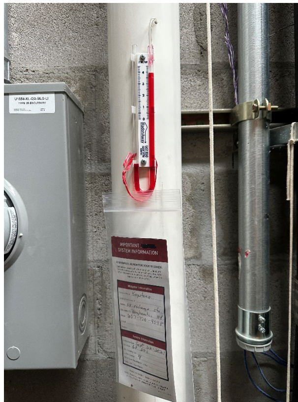
Photograph 4: View of the u-tube reading from the GP-501 fan.
