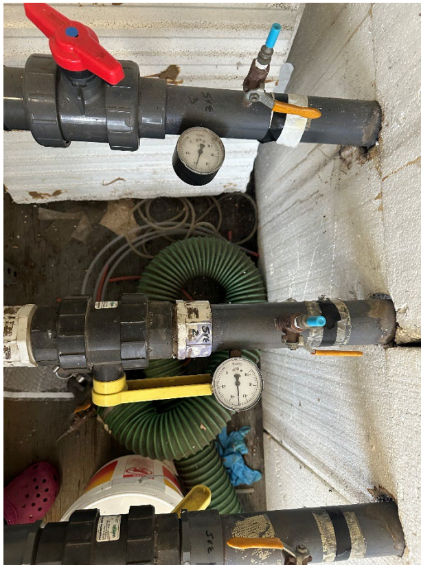
Photograph 1: View of the SSDS vacuum gauges.
