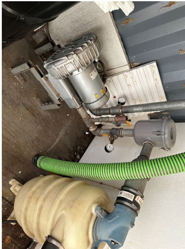
Photograph 6: View of the blower and knockout tank.
