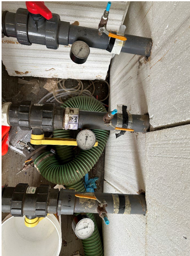
Photograph 1: View of the SSDS vacuum gauges.
