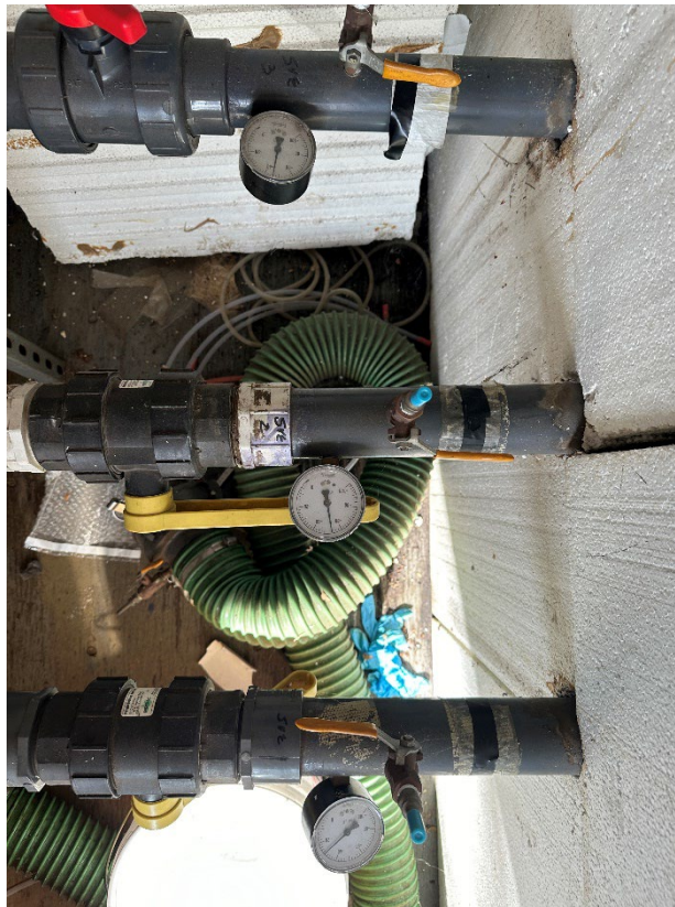
Photograph 1: View of the SSDS vacuum gauges.
