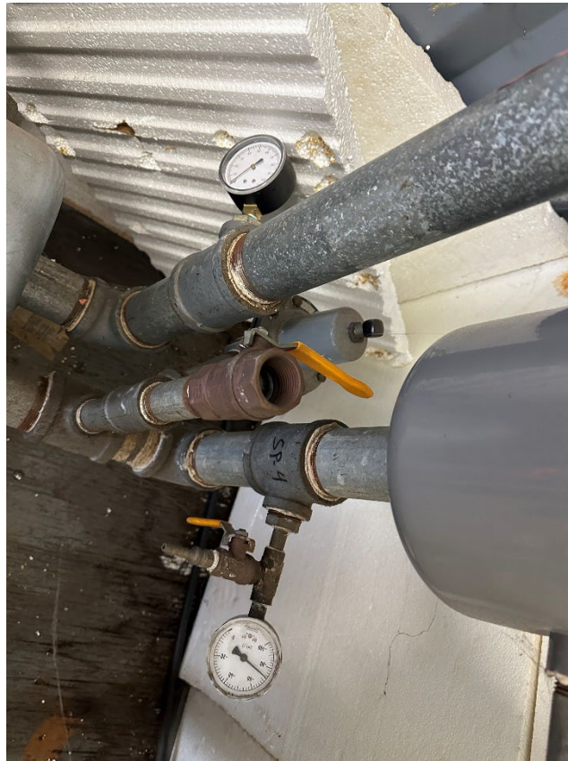
Photograph 5: View of the blower vacuum gauge.
