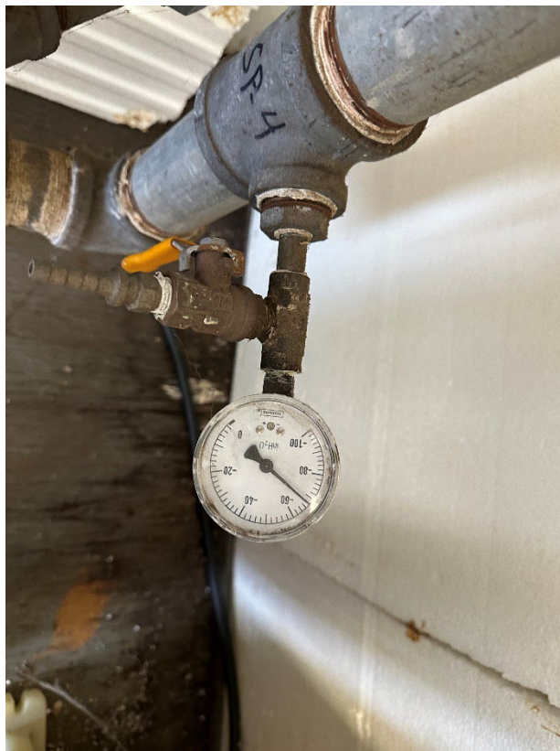
Photograph 2: View of the blower vacuum gauge.
