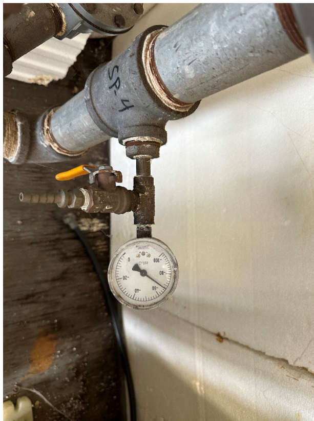
Photograph 2: View of the blower vacuum gauge.
