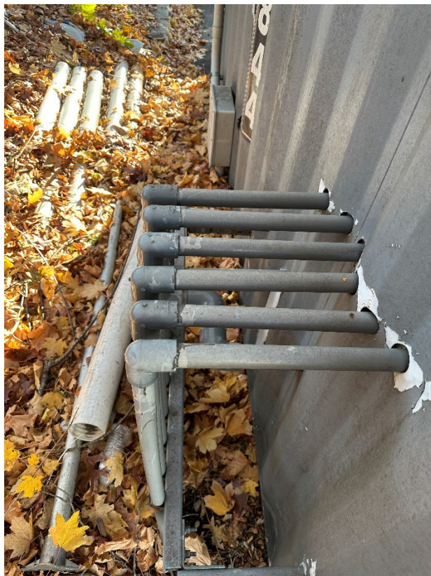
Photograph 2: View of the exterior piping associated with the monitoring points.
