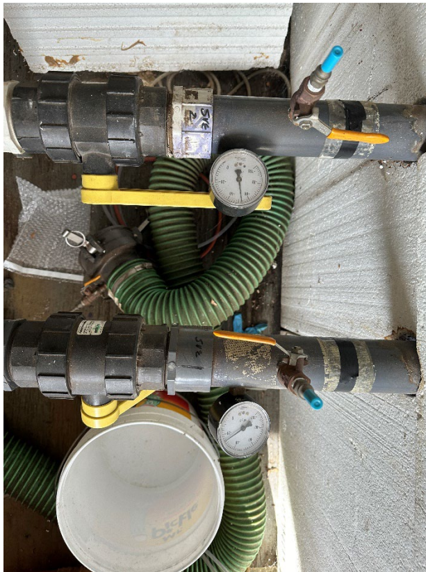
Photograph 1: View of the SSDS vacuum gauges.
