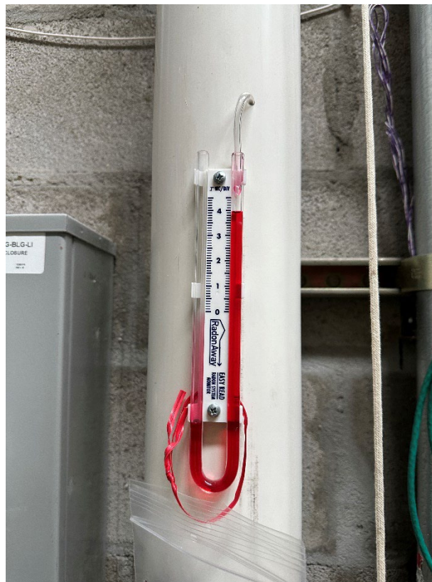
Photograph 4: View of the u-tube reading associated with the GP-501 fan.
