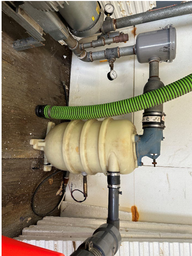
Photograph 3: View of the knockout tank.
