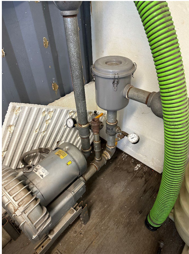
Photograph 3: View of the blower.
