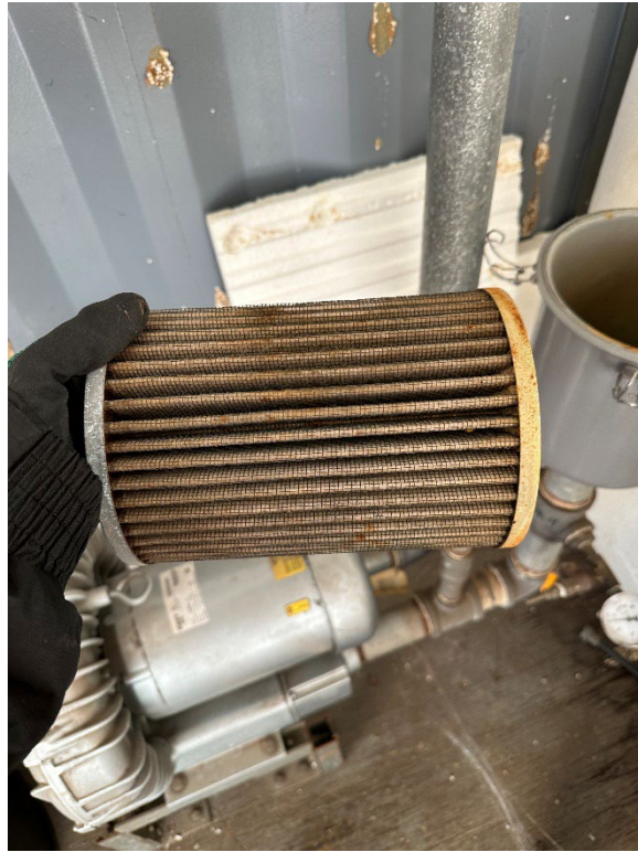
Photograph 5: View of the air filter from the blower.
