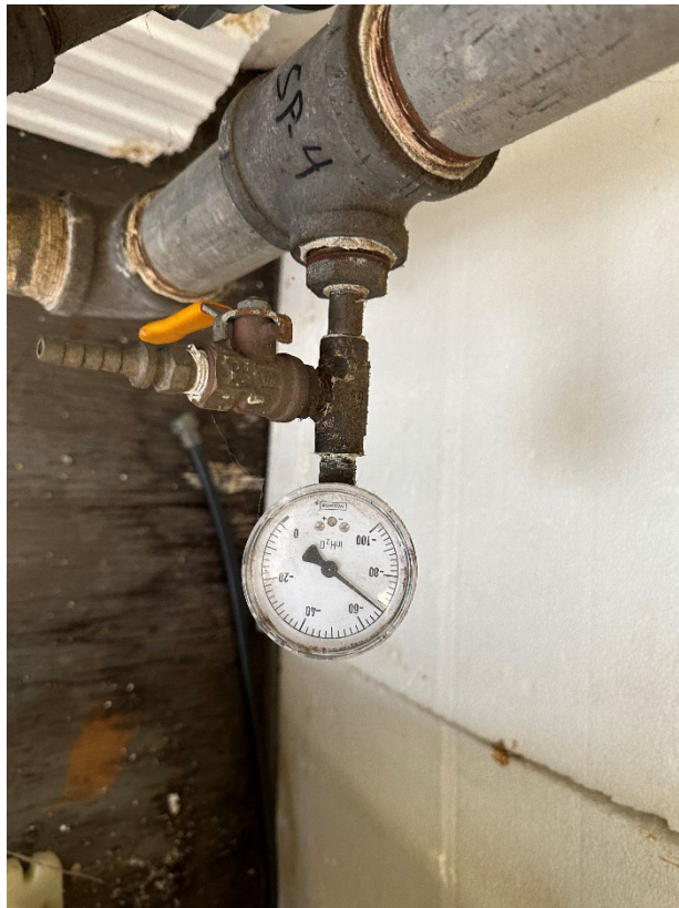
Photograph 2: View of the blower vacuum gauge.
