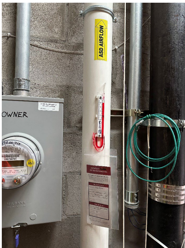
Photograph 5: View of the u-tube reading from the GP-501 fan.
