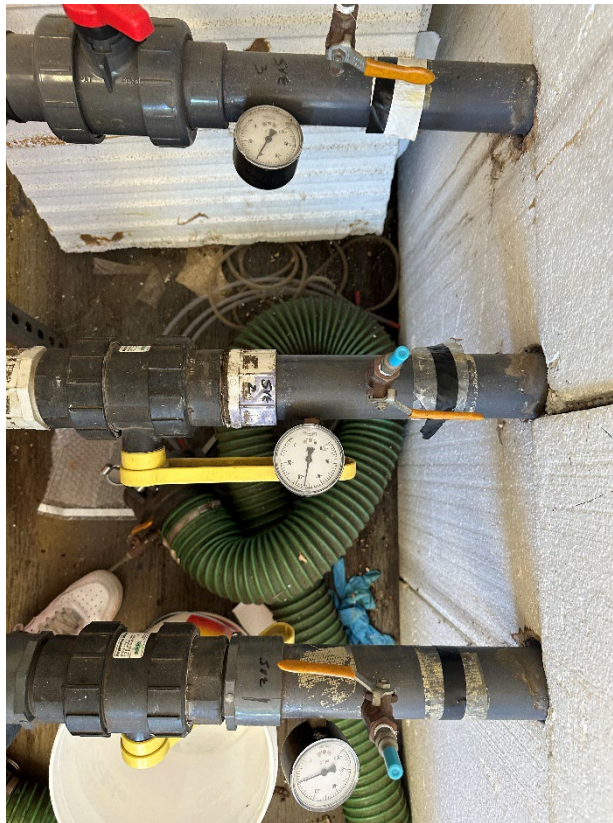
Photograph 1: View of the SSDS vacuum gauges.
