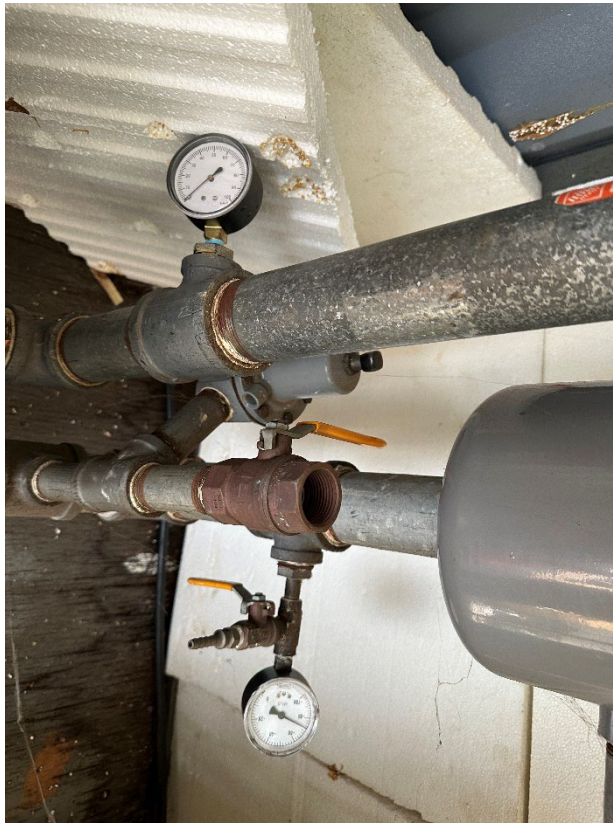
Photograph 3: View of the blower vacuum gauge.
