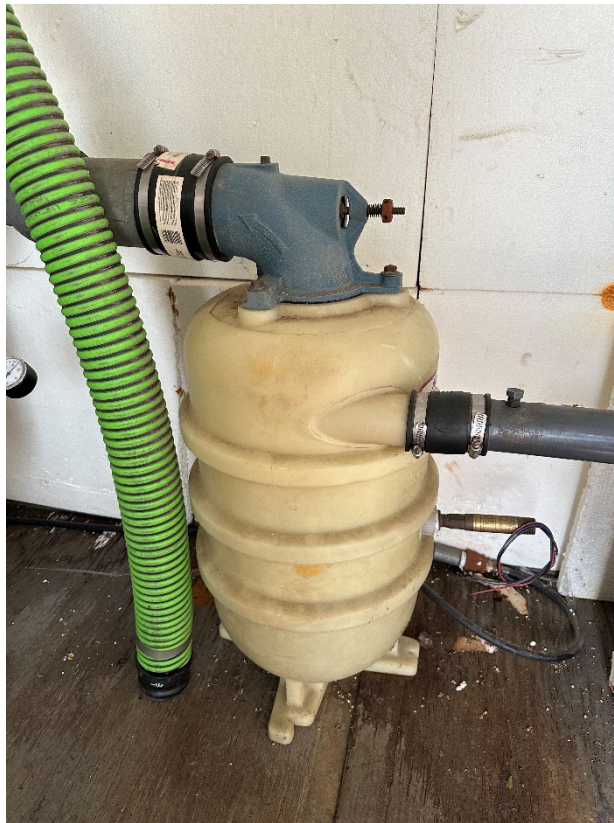
Photograph 1: View of the knockout tank.
