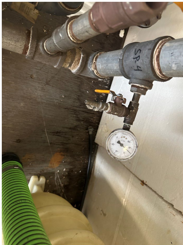
Photograph 2: View of the blower vacuum gauge.
