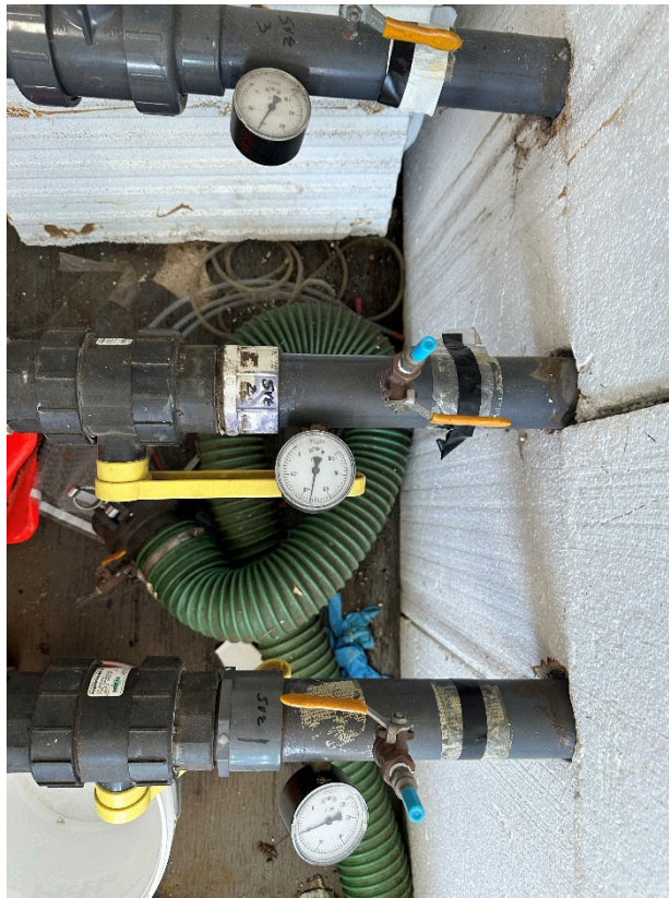
Photograph 1: View of the SSDS vacuum gauges.
