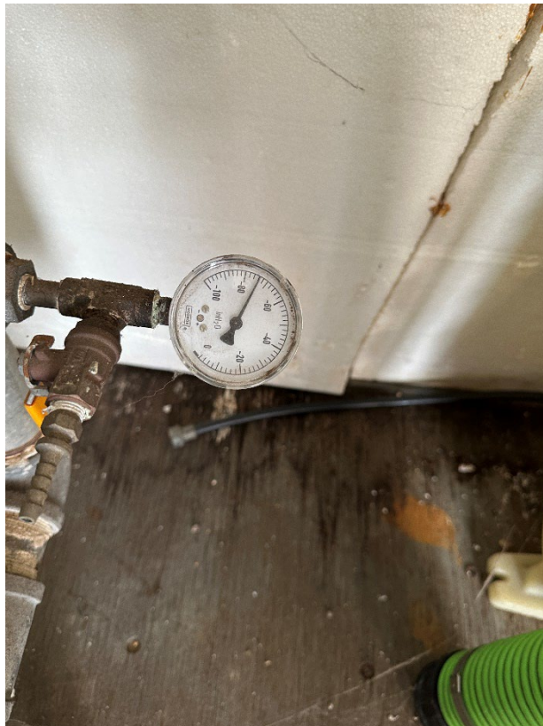
Photograph 2: View of the blower vacuum gauge.
