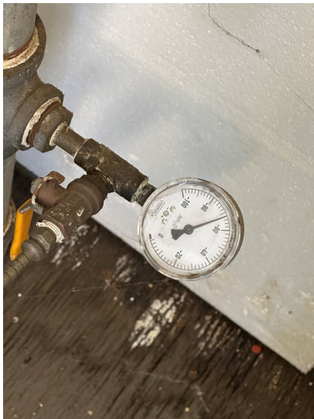
Photograph 2: View of the blower vacuum gauge.
