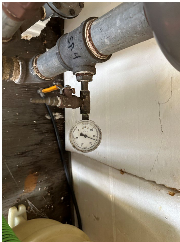
Photograph 2: View of the blower vacuum gauge.
