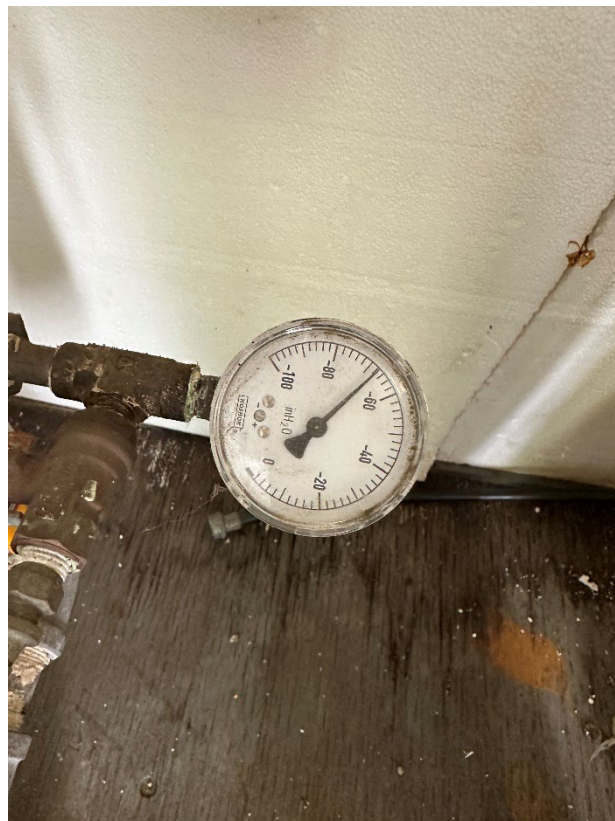
Photograph 2: View of the blower vacuum gauge.
