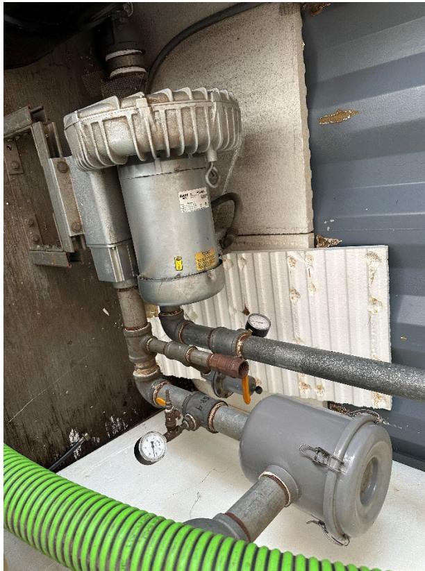
Photograph 3: View of the blower.
