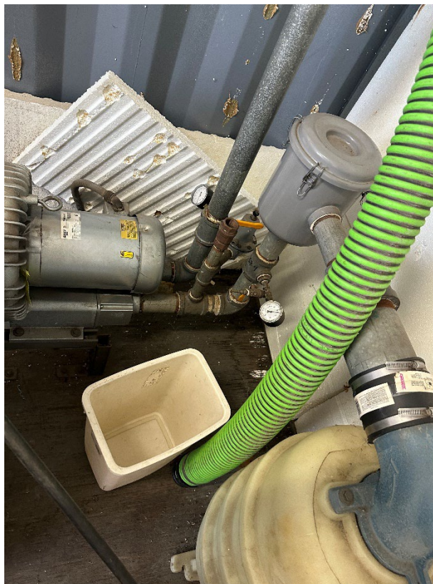
Photograph 4: View of the blower and interior piping.
