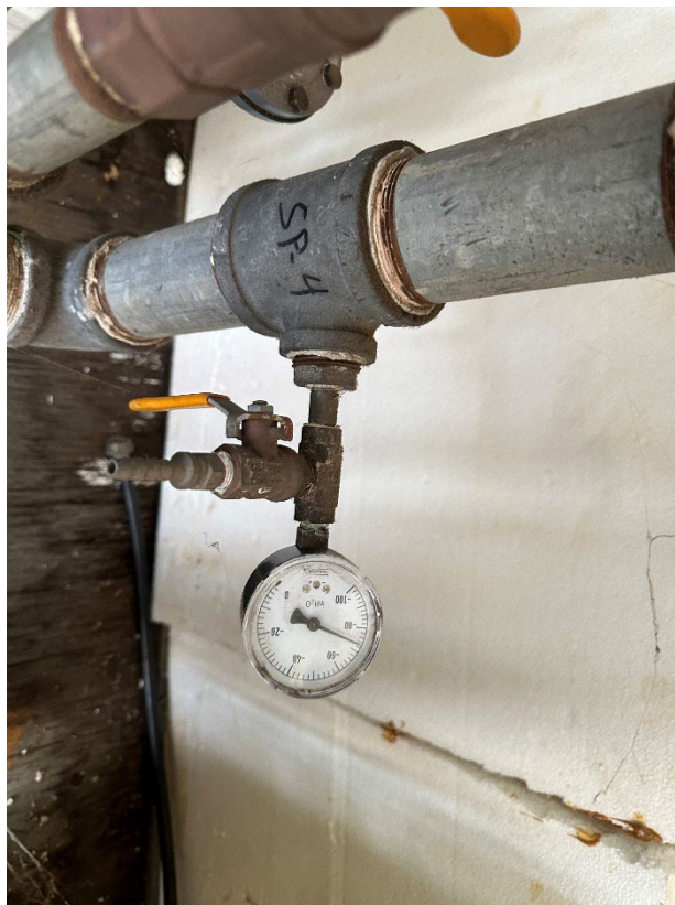
Photograph 2: View of the blower vacuum gauge.
