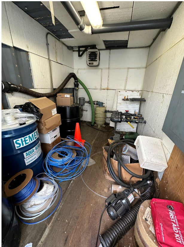
Photograph 1: View inside of the SSDS trailer.
