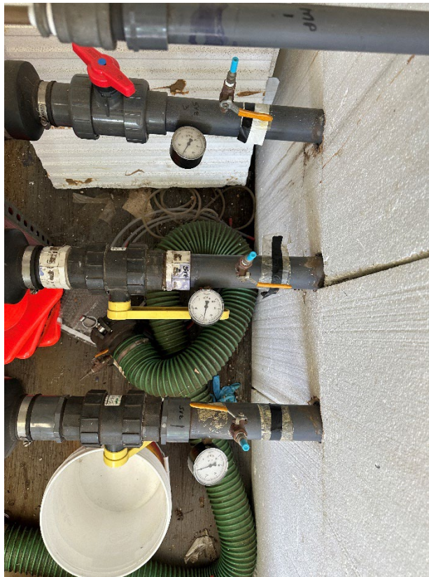
Photograph 1: View of the SSDS vacuum gauges.
