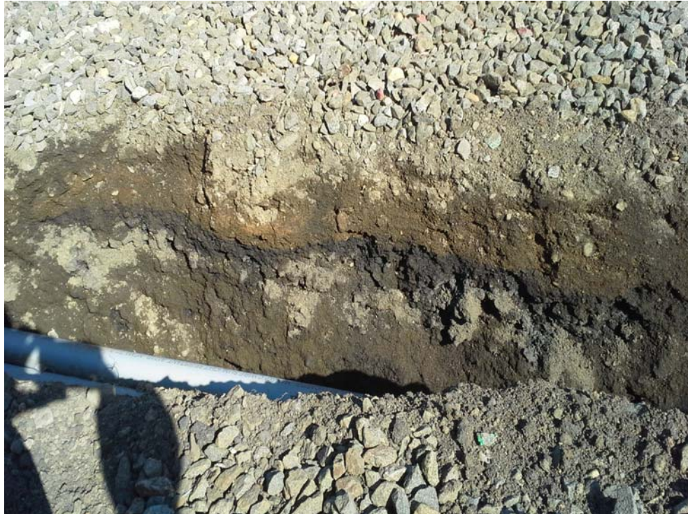
Photo 4: Coal clinker observed within cable trench excavation.
