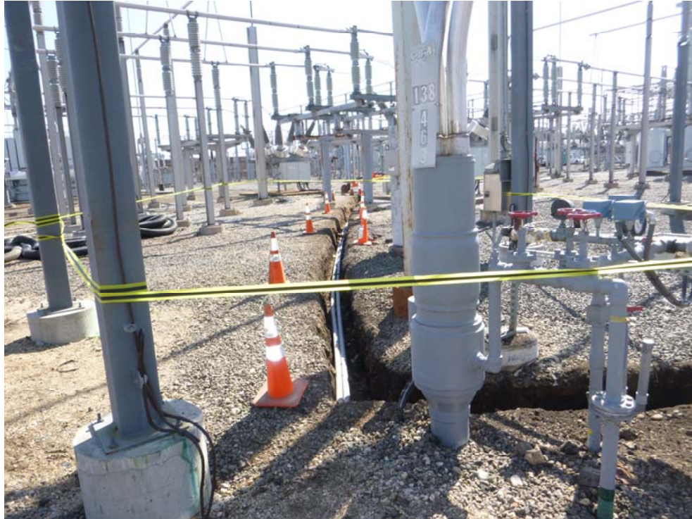
Photo 6: View of the northeast cable trench excavation with the area properly secured.
