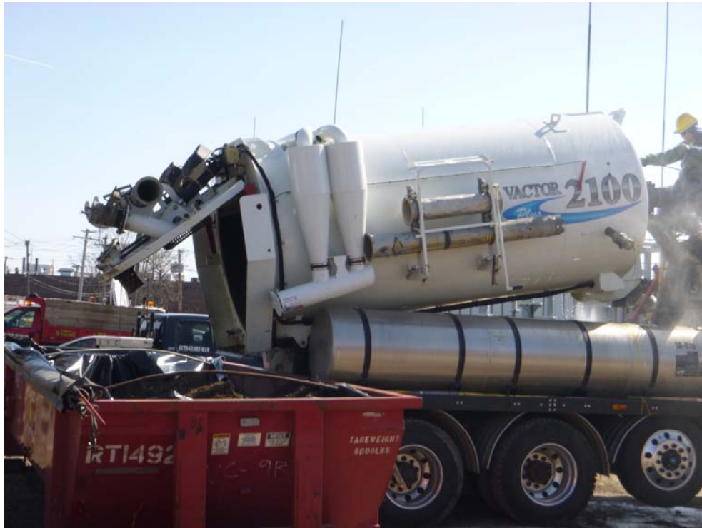
Photo 5: Guzzler truck dumping soil from cable trench excavation into a lined roll off.
