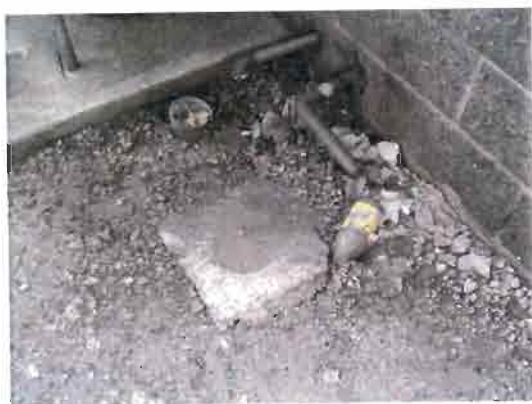
3. Location of MW-1 and boiler blow-down discharge piping in yard area.
