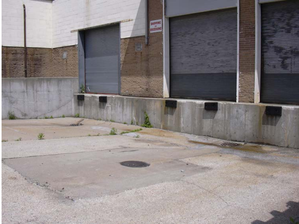
Photo 11: Loading area. Rear of building. Note: Storm drain.
