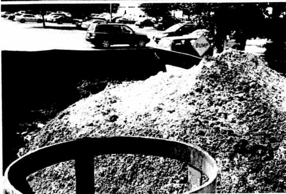
Photo 13: Sediment From Leaching Pool
