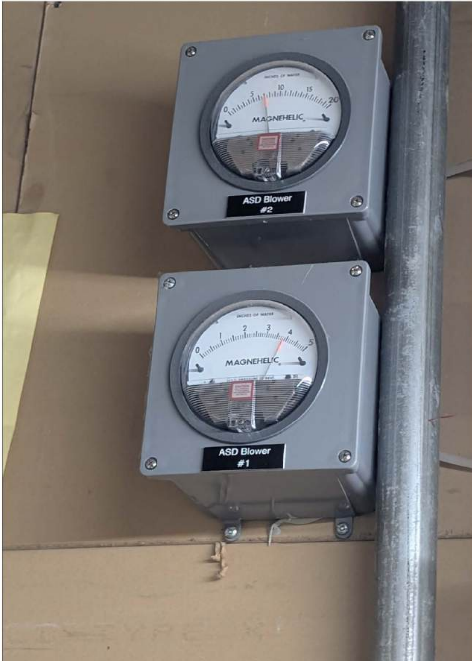
SSDS #1 & #2 Gauges and Alarms in Rear Office
