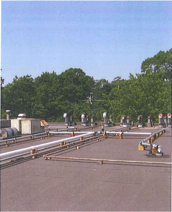
Duct work on roof
