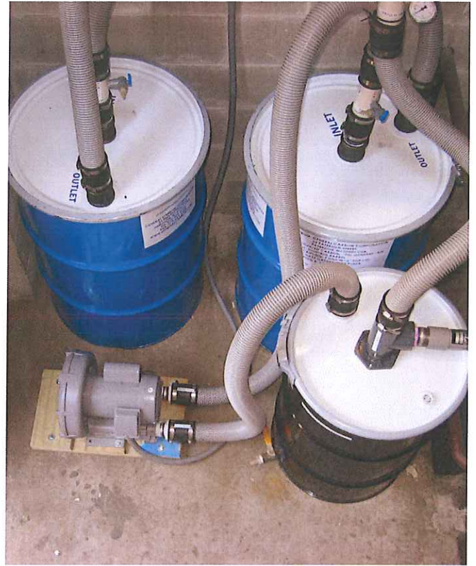
SSD blower and drums
