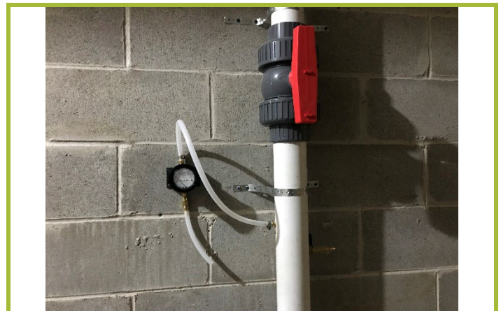
Photo #6: Typical riser with ball valve and vacuum gauge.
