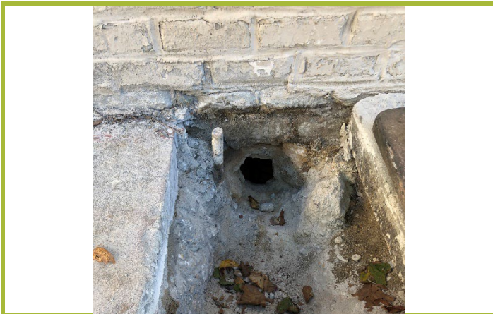
Photo #3: Basement penetration for riser to roof.
