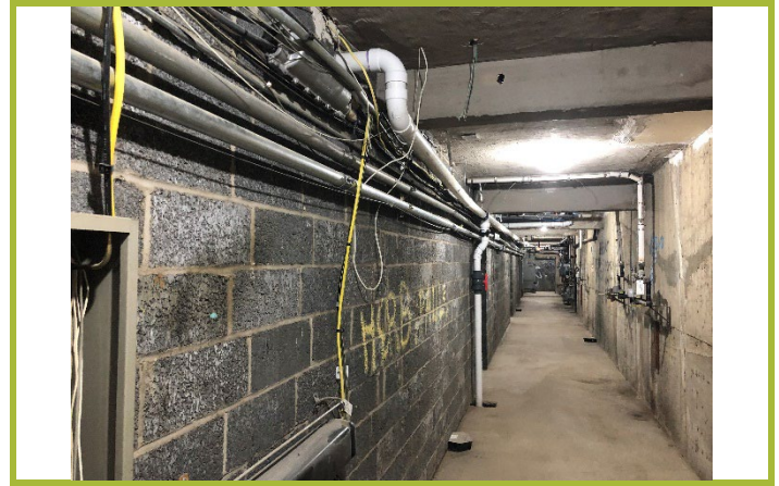
Photo #2: Typical riser with valve and piping run.
