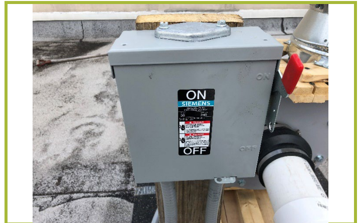
Photo #10: Blower local disconnect switch.
