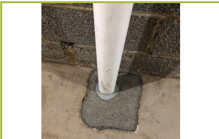
Photo #5: Typical riser with cement seal.
