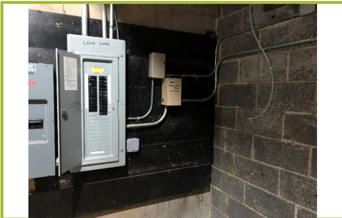
Photo #9: Landlord electrical panel.
