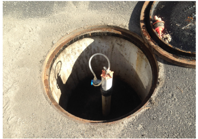
Exterior SVE well capped for pilot test.
