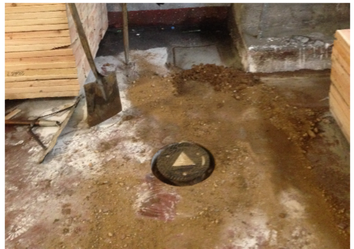
View of interior sub-slab vent (SVE-6).
