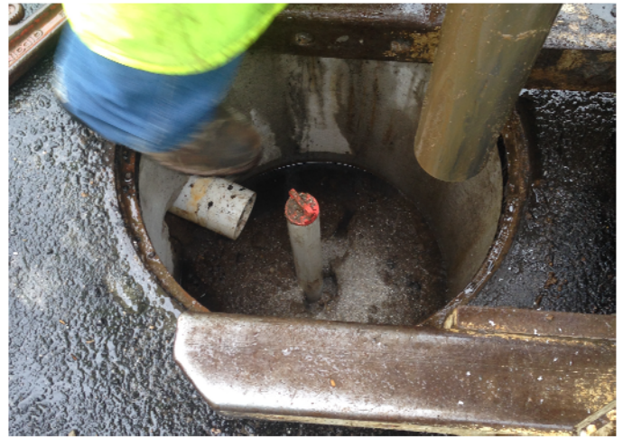
View of exterior SVE well.
