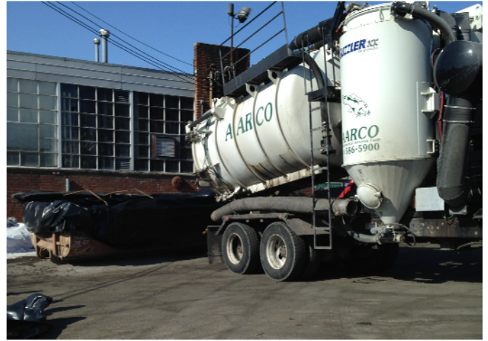
View of guzzler unloading material from within the cesspool into a hazardous waste roll off.
