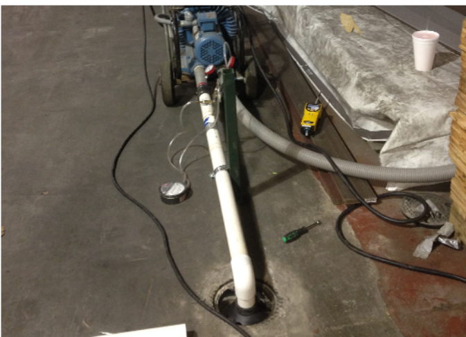
View of blower attached to interior sub-slab vent (SVE-5) during pilot test.
