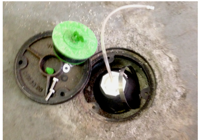
Interior sub-slab vent capped for pilot test.
