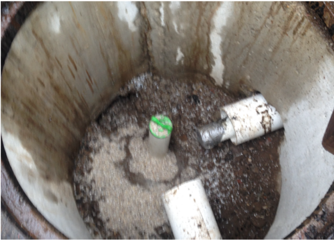
View of exterior SVE well.
