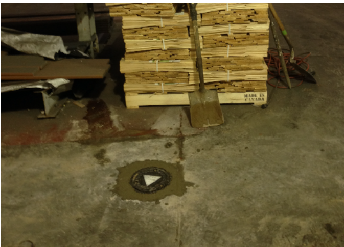
View of interior sub-slab vent (SVE-5).
