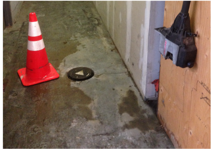
View of interior sub-slab vent (SVE-4).
