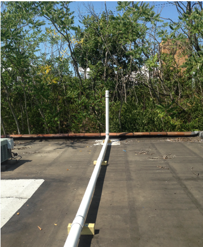
View of venting system layout on the roof.
