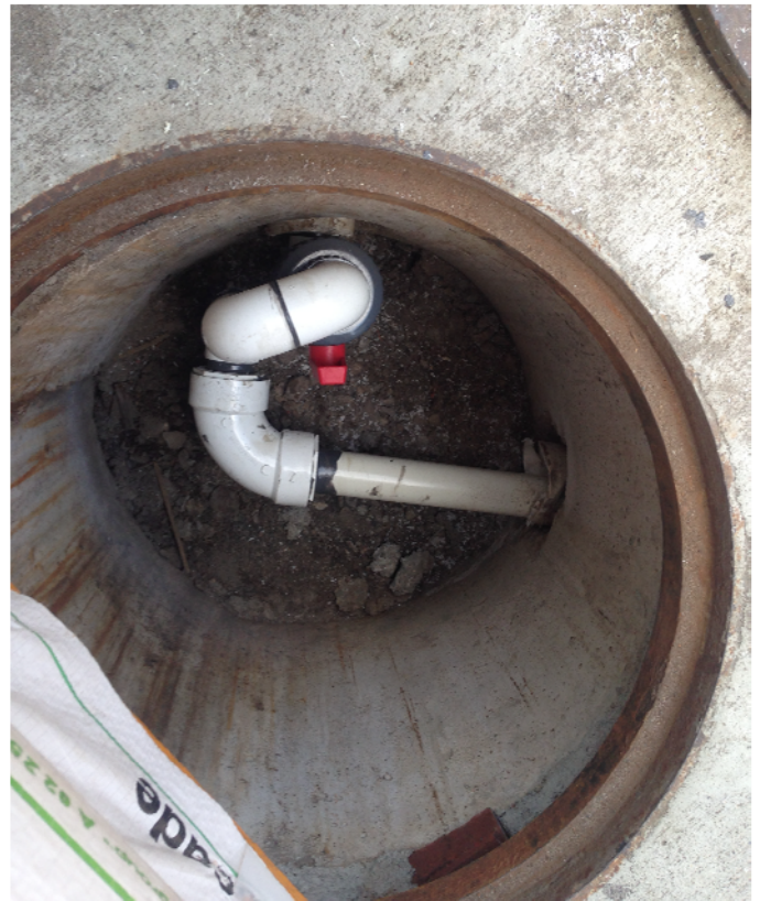
Interior view of SVE well inside 24-inch manhole.
