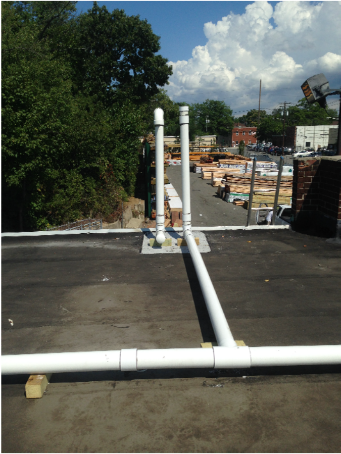
View of venting system layout on the roof.
