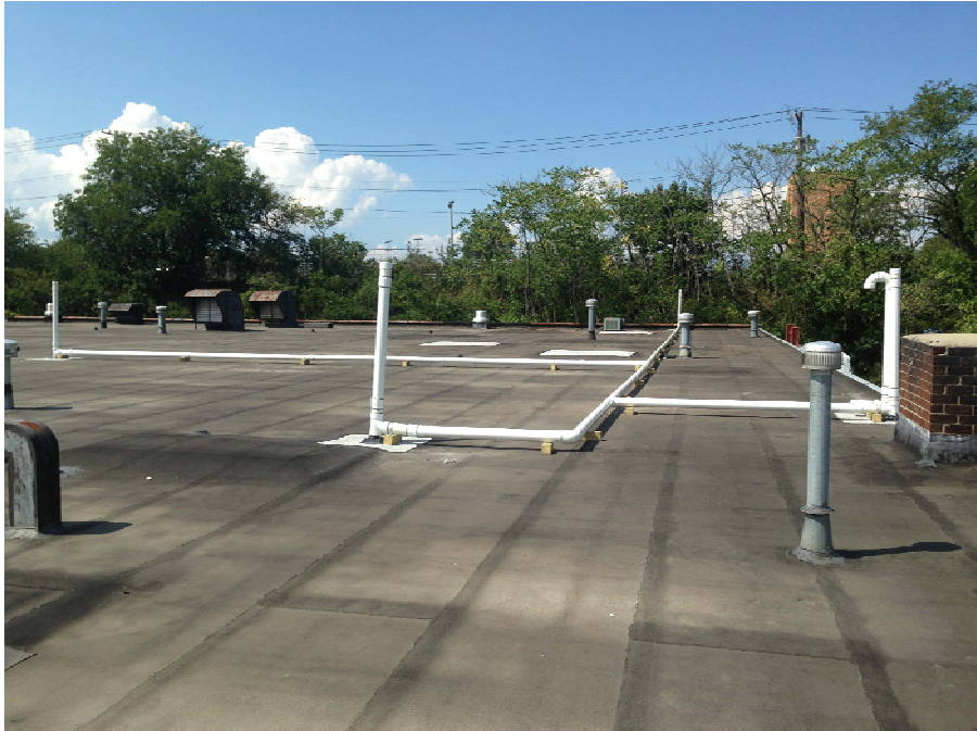
View of venting system layout on the roof.
