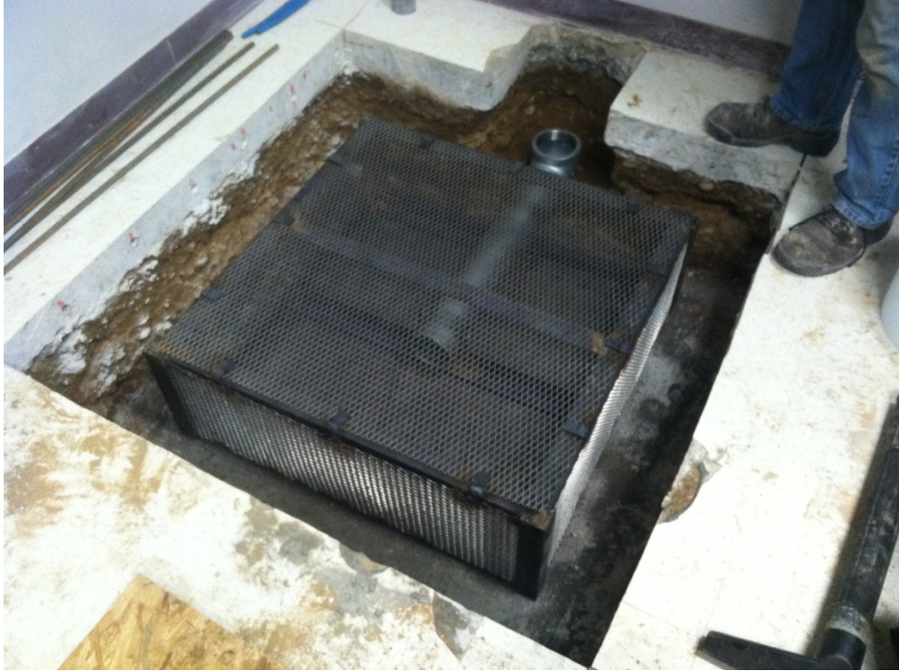
SSVM Pilot Pit with Expanded Metal Box.
