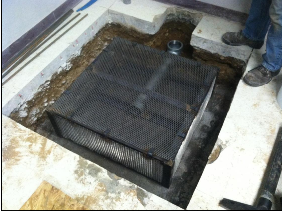
SSVM Suction Pit with Expanded Steel Cage
