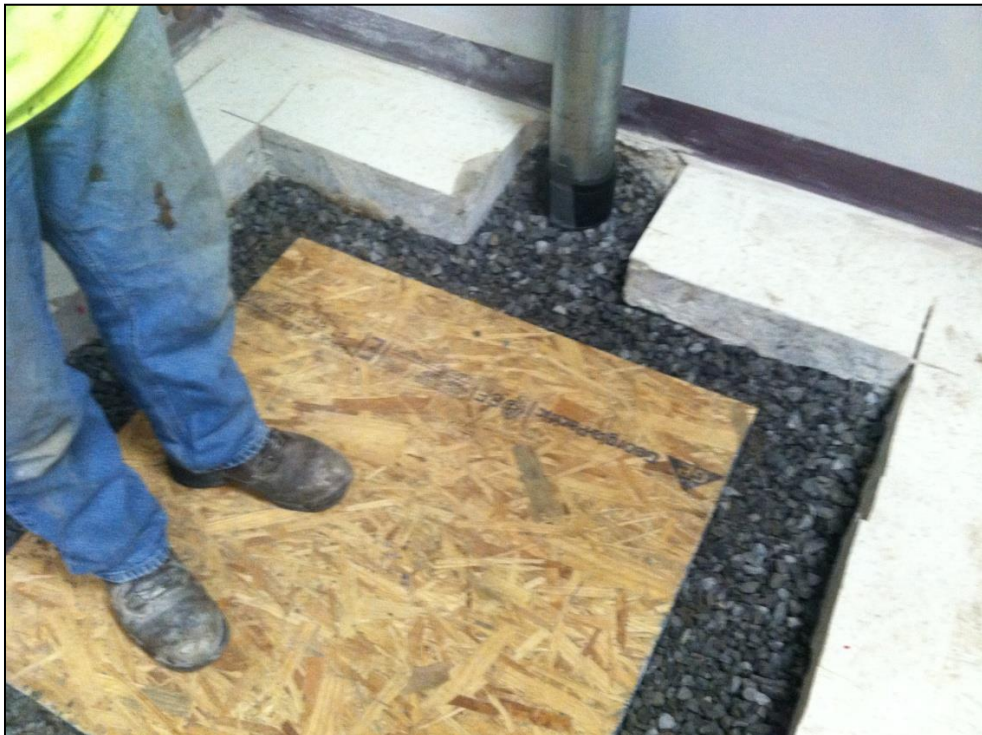
SSVM Suction Pit with Surrounding Stone
