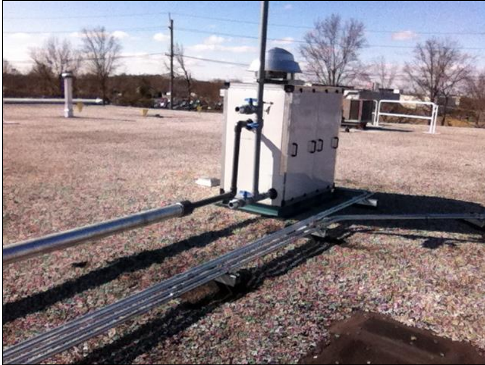
Blower #2 within Enclosure
