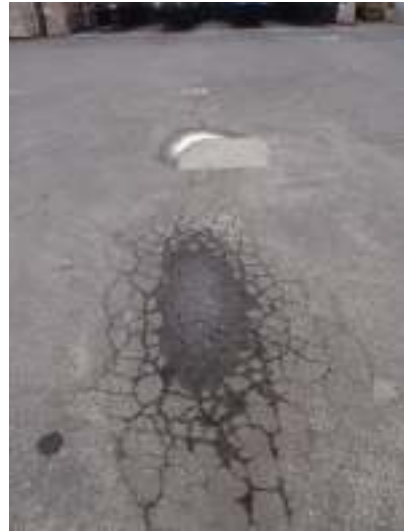
AOC—1: Detail of asphalt cracking in center of area. Looking west.
