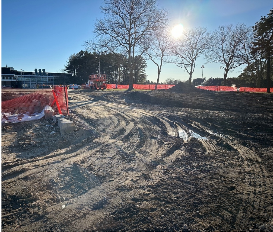
The one access point to the regulated work area on the south side of the site will be graded with RCA.
