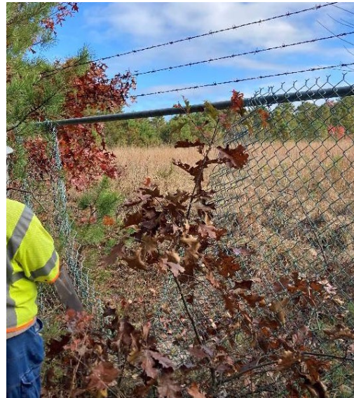
Photo 2: Hole in fencing leading to Capped Area.
