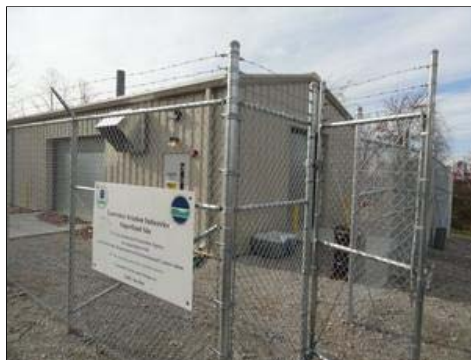
The EPA's on-site pump and treat plant at Lawrence Aviation will function nonstop for 20 years to remove carcinogens from the groundwater. Photos by D. Willinger. (click for larger version)
