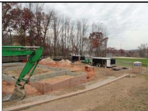
The foundation for the EPA's water treatment plant in Port Jefferson clearly shows the size of the facility's footprint. Caroline Avenue ball field is visible in the background. ( click for larger version )
