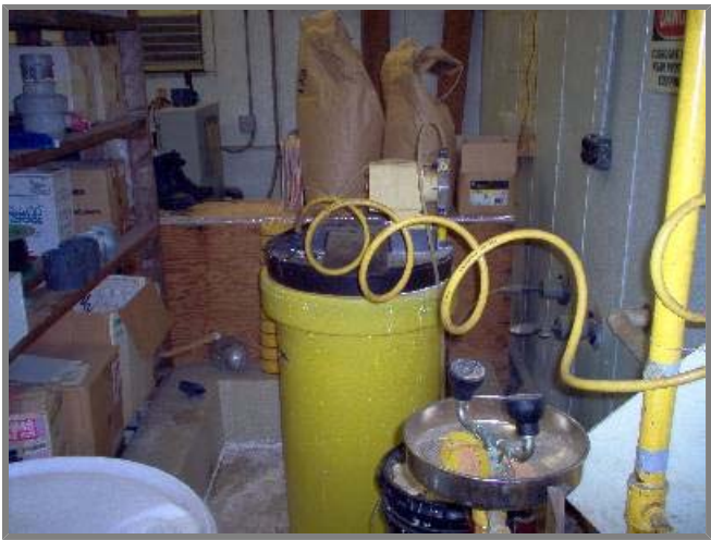
Photo left. Inside the treatment plant.
