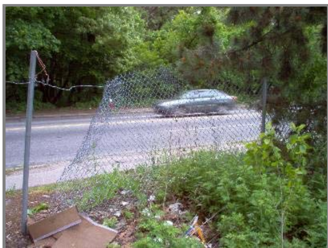
Photo left. Liberty Industrial site, broken gate.
