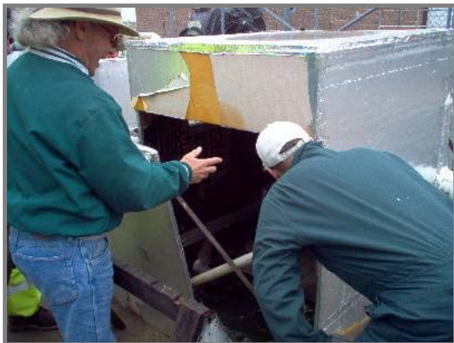
Photo left. Looking into one of the insulated boxes in the treatment compound. Kenn has thoroughly insulated all outdoor piping and pumps that might be prone to freezing. This box is placed over the sump pump and has a heater as well.
