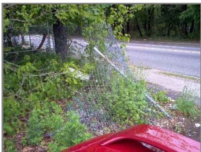
Photo left. Liberty Industrial site, broken gate.
