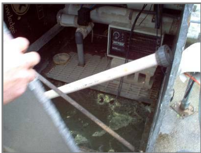
Photo left. A closer look at the heater.
