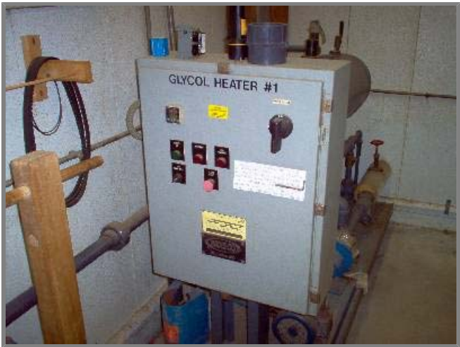
Photo left. View of the "glycol heater." This unit warms the air discharging from the airstripper before it enters the carbon filters.
