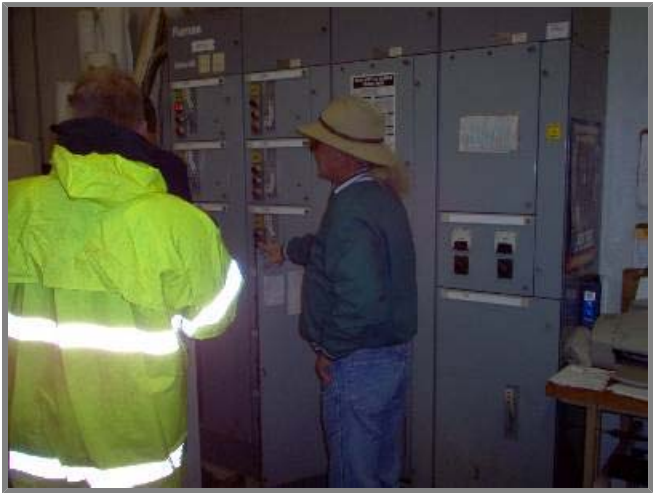
Photo left. Inside the treatment plant.
