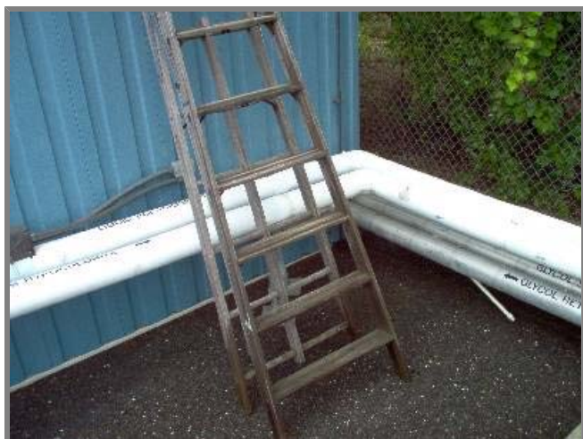
Photo left. Exterior influent/effluent piping.
