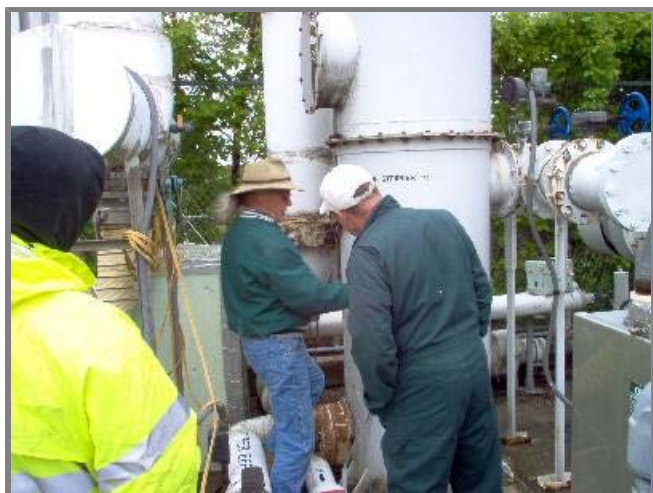
Photo left. Base of the airstripping tower.
