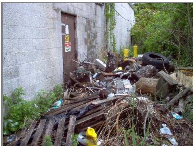
Photo left. NYSDEC-owned plant at Site No. 152077, ServAll Laundry, 8 Drayton Avenue, Bayshore, NY 11706. We wish to dismantle this plant. The first step in decommissioning would be garbage removal! We couldn't gain access through the door on 5/26-- our key didn't work plus debris was piled deep against the door.
