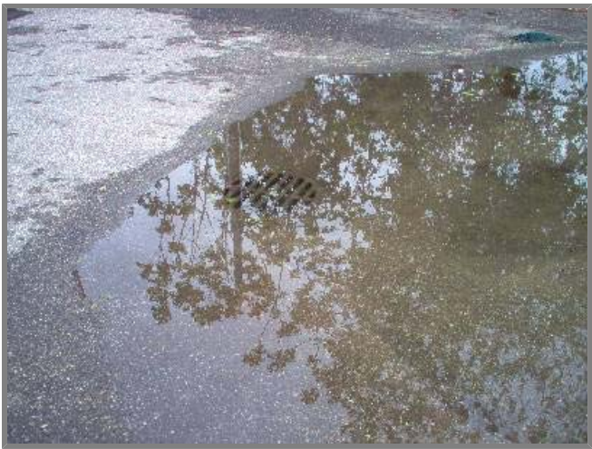
Photo left. Plugged drain in front of the plant.
