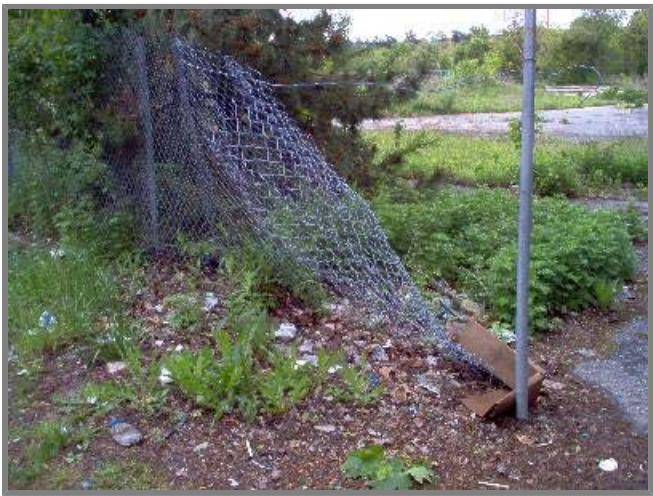
Photo left. Liberty Industrial site, broken gate.
