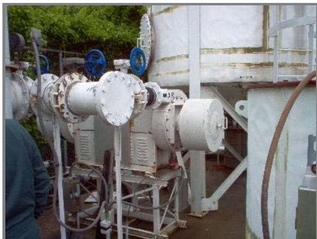
Photo left. These blowers force air up through the packed column of the airstripper.
