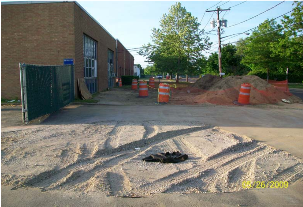
100_00677.jpg - Completed PDS-5, 51 Cabot St.
