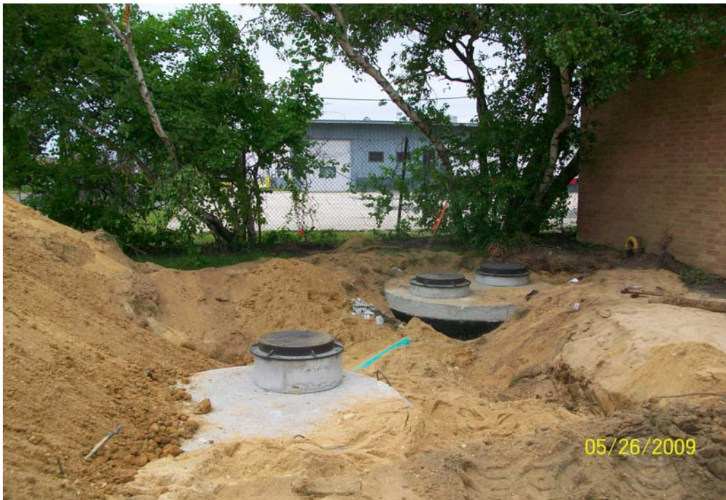
100_00691.jpg - PCP-2A and piping installed to PST-2, 61 Cabot St.
