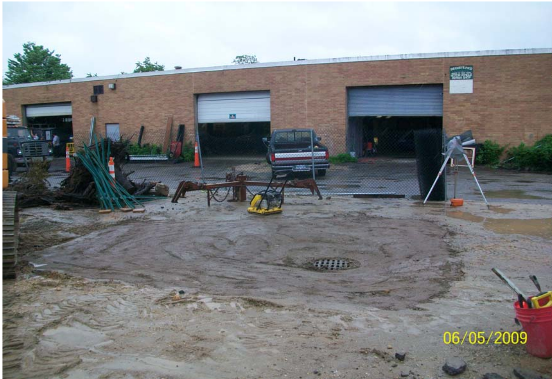
100_0769.jpg - PDS-12, 50 Dale St., completely installed
