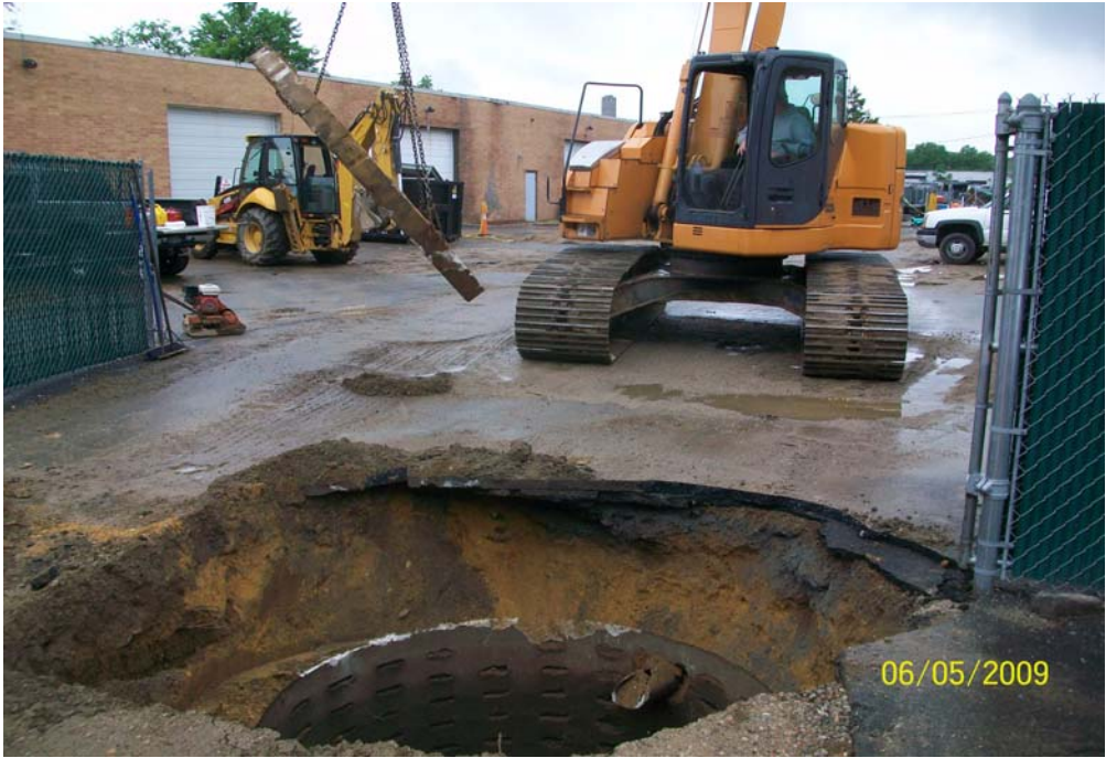
100_0762.jpg - CP-1, 51 Cabot St., partially abandoned
