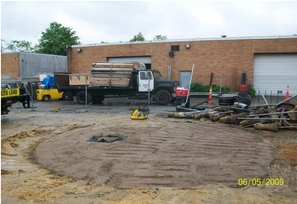
100_0767.jpg - PDS-11, 50 Dale St., completely installed
