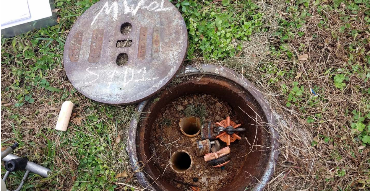
Photograph 9: Monitoring well manhole containing MW-01S & MW-01D1.
