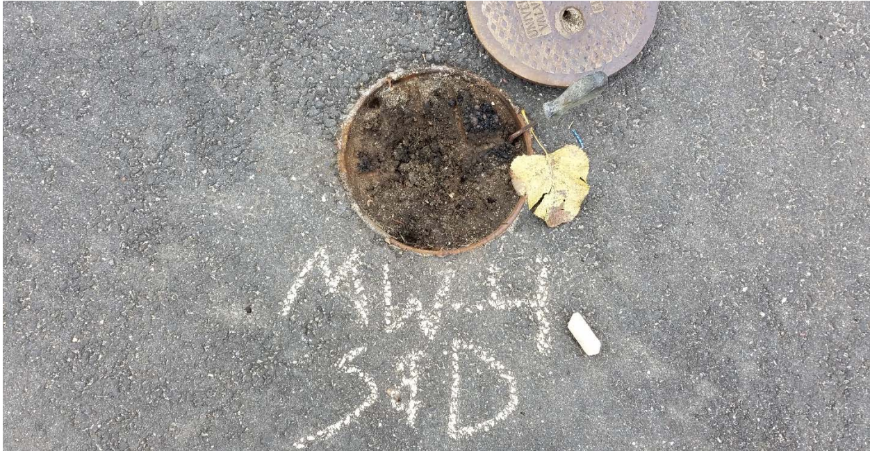
Photograph 11: Monitoring well manhole containing MW-04S & MW-04D. Asphalt cleared from casing prior to sampling event.
