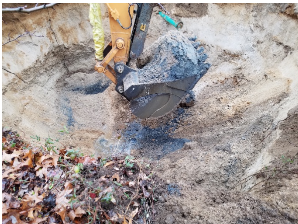
SB-22 viewed to the west. Grey impacted soils visible on the bottom of the excavation at approximately 5'-7'.
