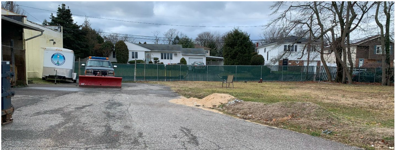
Above: View of part of the back of the industrial building (at left) at the subject property looking west. The asphalt pavement cover over the former LP-1 area was observed to be in good condition throughout the covered area. The small pile of sand (at center, not in the covered area) is used on the parking and driveway areas during snow and ice conditions. Well MW-1, which is upgradient of the capped area and protected by a steel standpipe, is visible in the right background.
