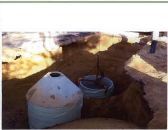
Photo #3 – View of the installation of the new leaching pools. LP-2R is shown on the left, LP-3R is being installed on the right.
