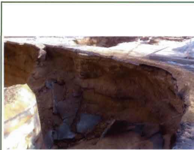
Photo #4 – View of the excavation for LP-1R (shown on the left). The excavation for LP-2 can be seen in the background.
