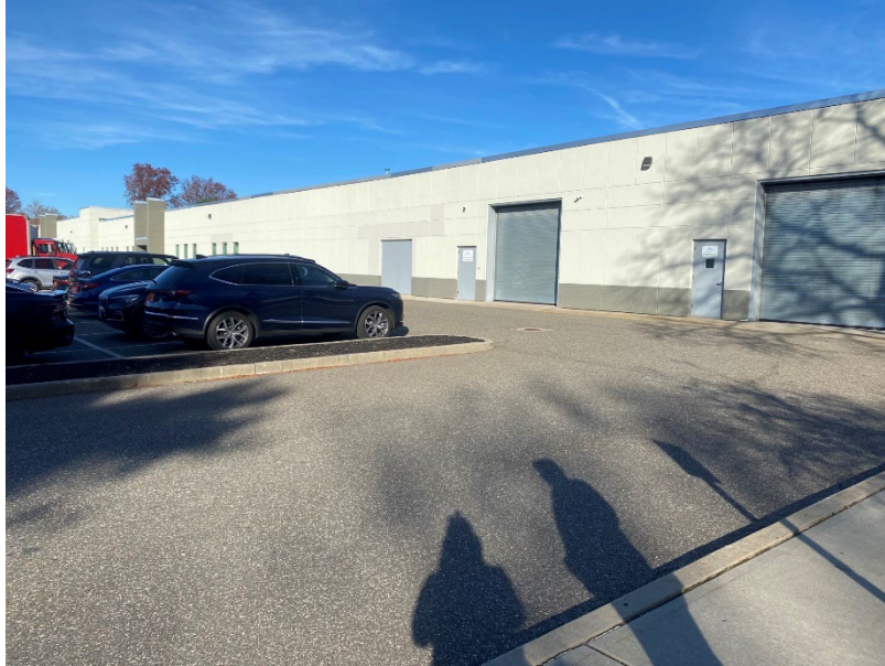
Above: Intact pavement showing no new disturbances above cover over former leaching pools LP-1 and LP-2.
