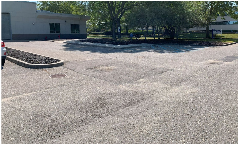
Above at top left: Intact pavement over the cover on top of former leaching pools LP-1 and LP-2. No cover disturbance was observed or reported.
