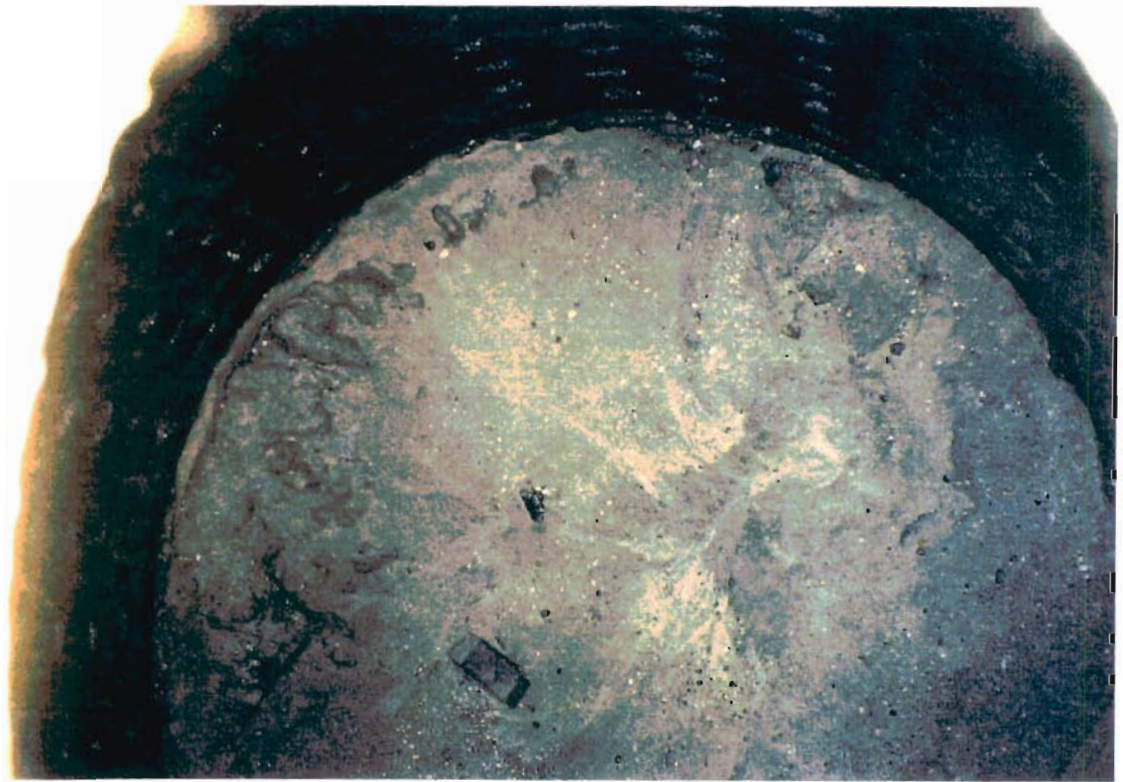
SANITARY OVERFLOW AFTER CLEANOUT
