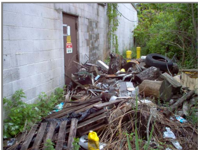
Photo left. NYSDEC-owned plant at Site No. 152077, ServAll Laundry, 8 Drayton Avenue, Bayshore, NY 11706. We wish to dismantle this plant. The first step in decommissioning would be garbage removal! We couldn't gain access on 5/26.
