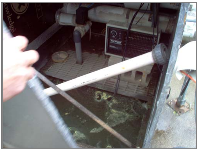
Photo left. Inside the treatment plant.
