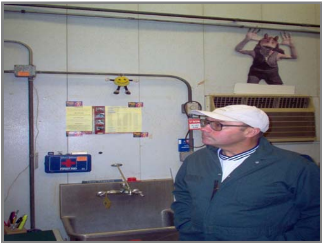
Photo left. Inside the treatment plant.
