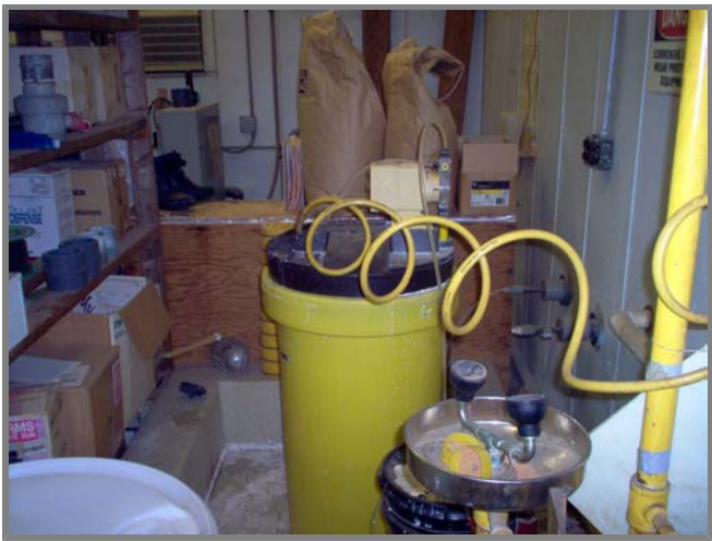
Photo left. Inside the treatment plant.
