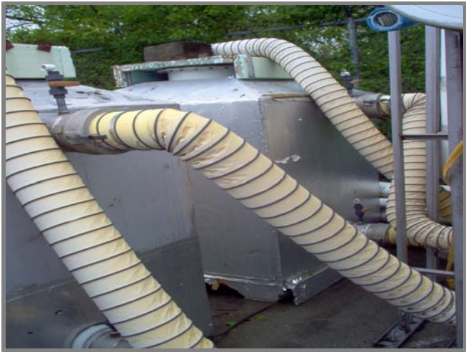
Photo left. Influent lines leading to the carbon vessels.
