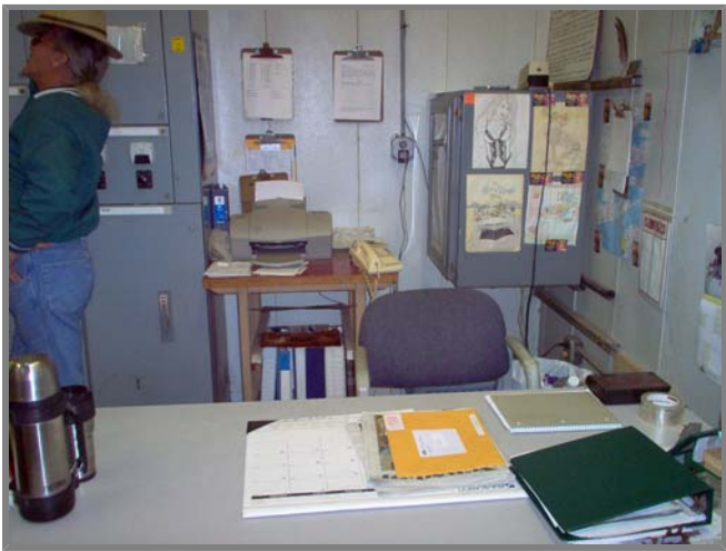
Photo left. Inside the treatment plant.
