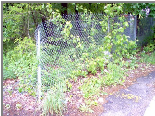
Photo left. Liberty Industrial site, broken gate.
