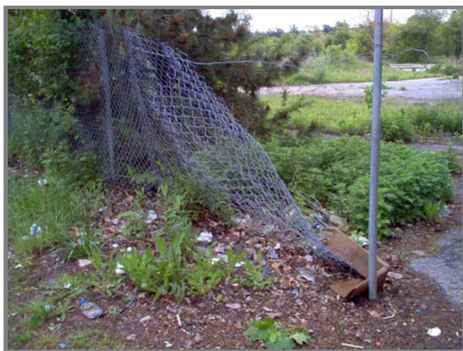
Photo left. Liberty Industrial site, broken gate.
