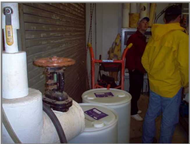
Photo left. Just inside the treatment plant.
