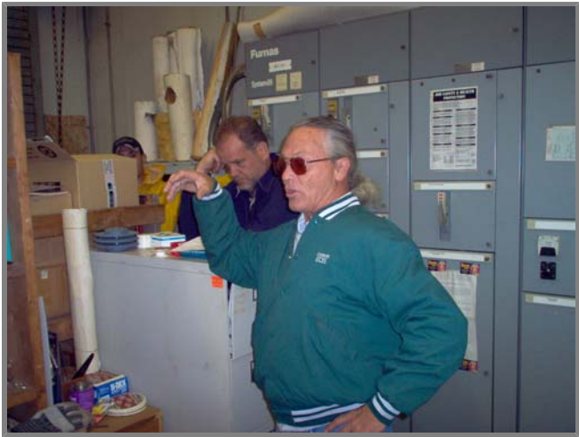
Photo left. Inside the treatment plant.
