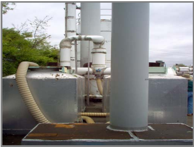
Photo left. Towers and tank. Descriptions from front to back: air discharge tower, air tower from top of air stripper to heater, air stripping tower, and water intake tank.
