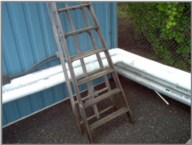
Photo left. Exterior piping.
