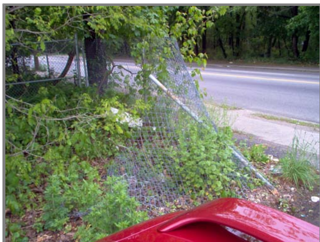
Photo left. Liberty Industrial site, broken gate.
