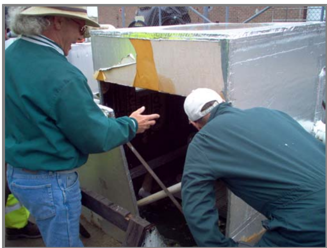
Photo left. Inside the treatment plant.
