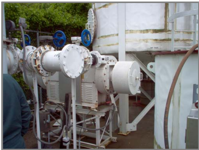
Photo left. Exterior piping.
