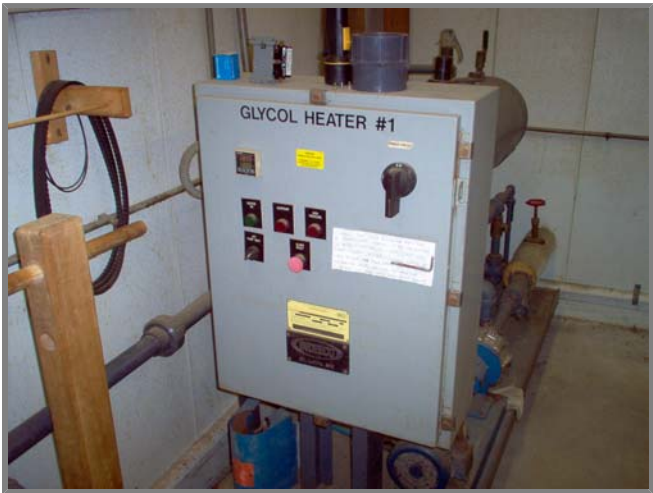
Photo left. Inside the treatment plant.
