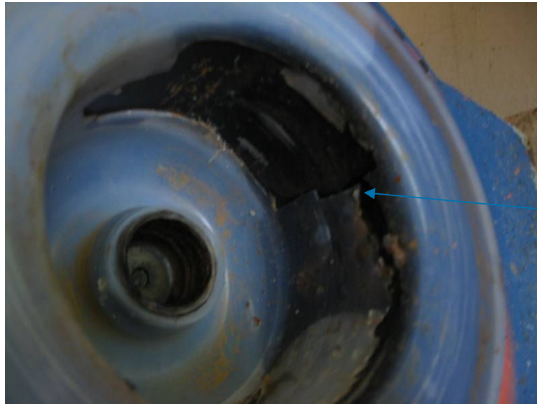
Damage to PFA Liner and Casing
