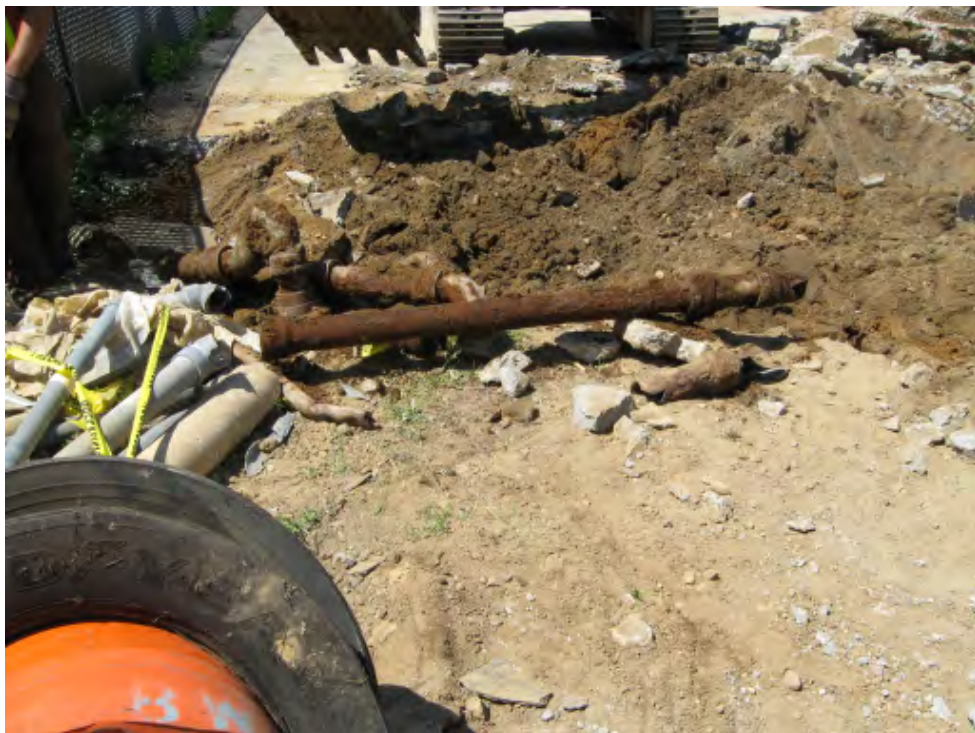
Photograph 16 – Excavation of below grade piping and drainage structures in the western portion of the site.
