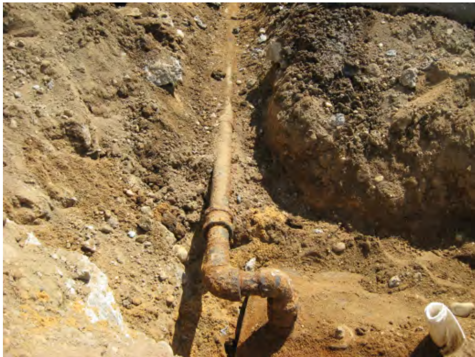
Photograph 8 – Wash Water UST, showing below grade piping, which connects to several below grade structures.
