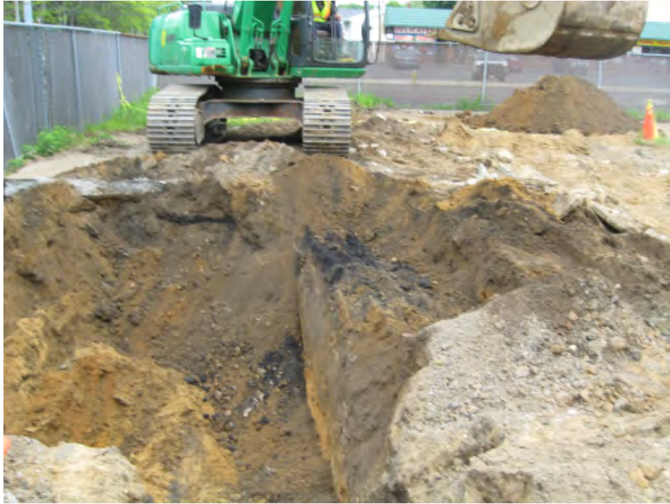
Photograph 15 – Excavation of soil in the western portion of the site, showing stained soil.
