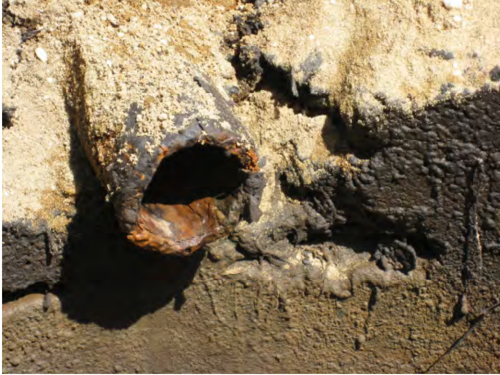
Photograph 19 – Close-up of westernmost identified dry well discharge piping.
