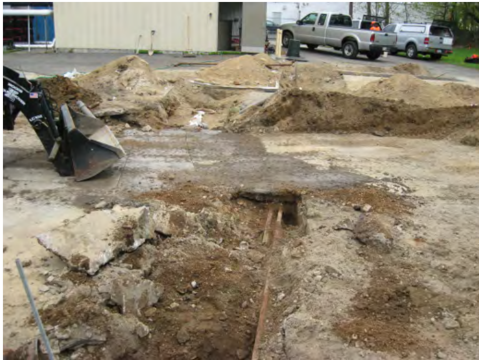
Photograph 12 – Below grade piping network, connecting to the westernmost dry well.
