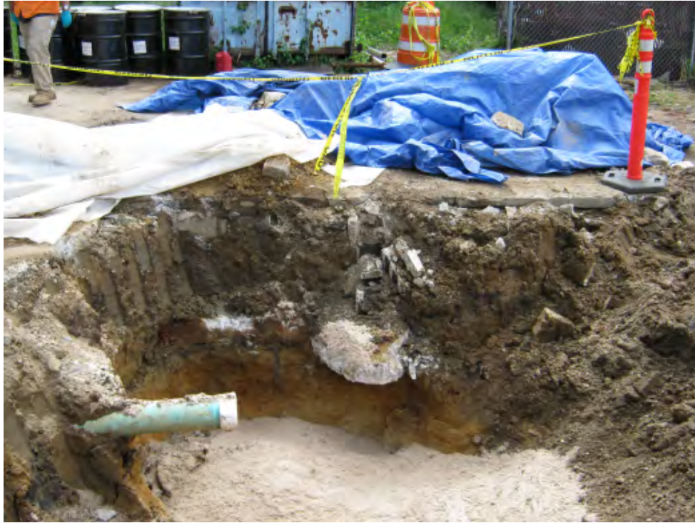
Photograph 11 – Below grade sewer pipe and southern portion of the overall UST excavation.
