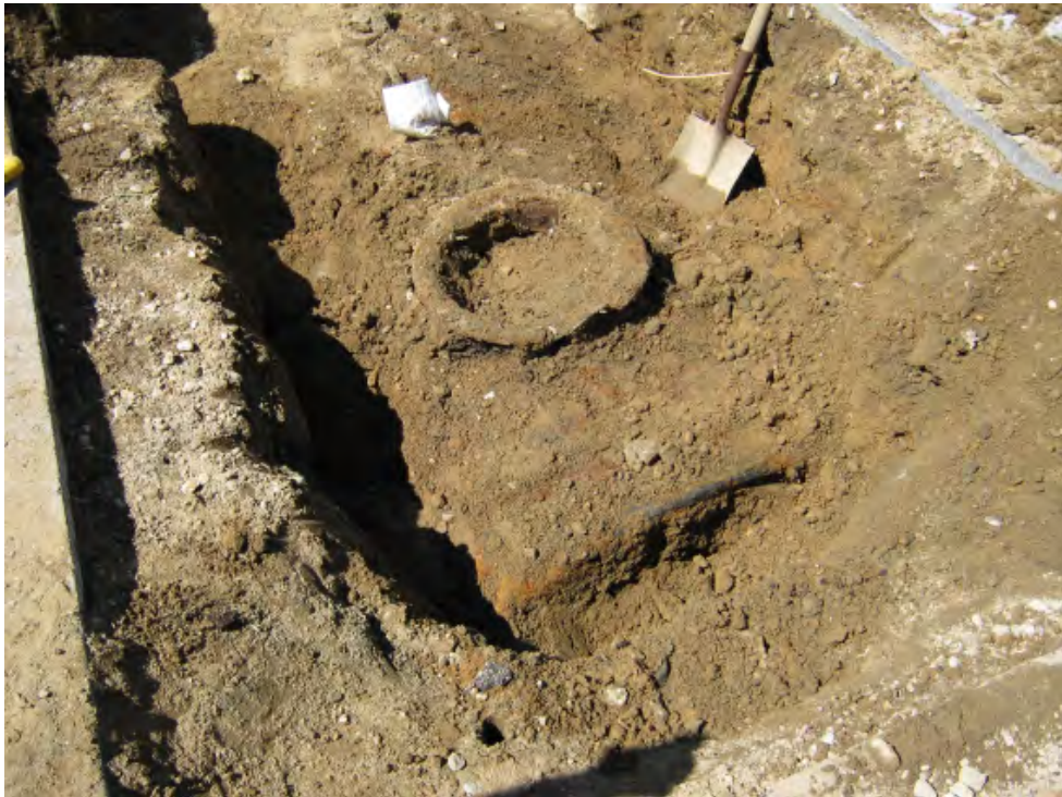
Photograph 4 – Exposed Wash Water UST.
