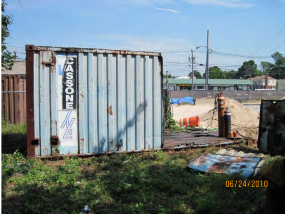
Photograph 29 – Sea container during demolition and removal, showing clean fill installation in the background.
