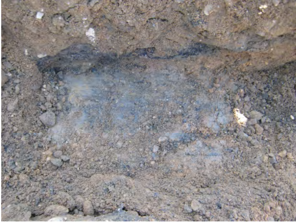
Photograph 5 – Area of stained soil in association with the Fuel Oil UST.
