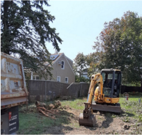
Fence damaged by the tree, south side
