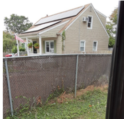
Fence damaged by tree after repairs, south side
