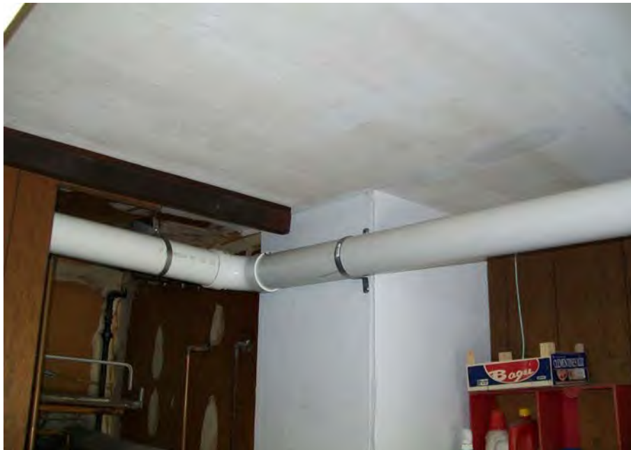
4. Suction piping, looking southeast toward boiler from central portion of garage
