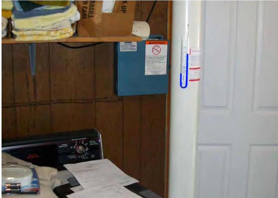
3. U-tube manometer installed on suction piping above SP-1
