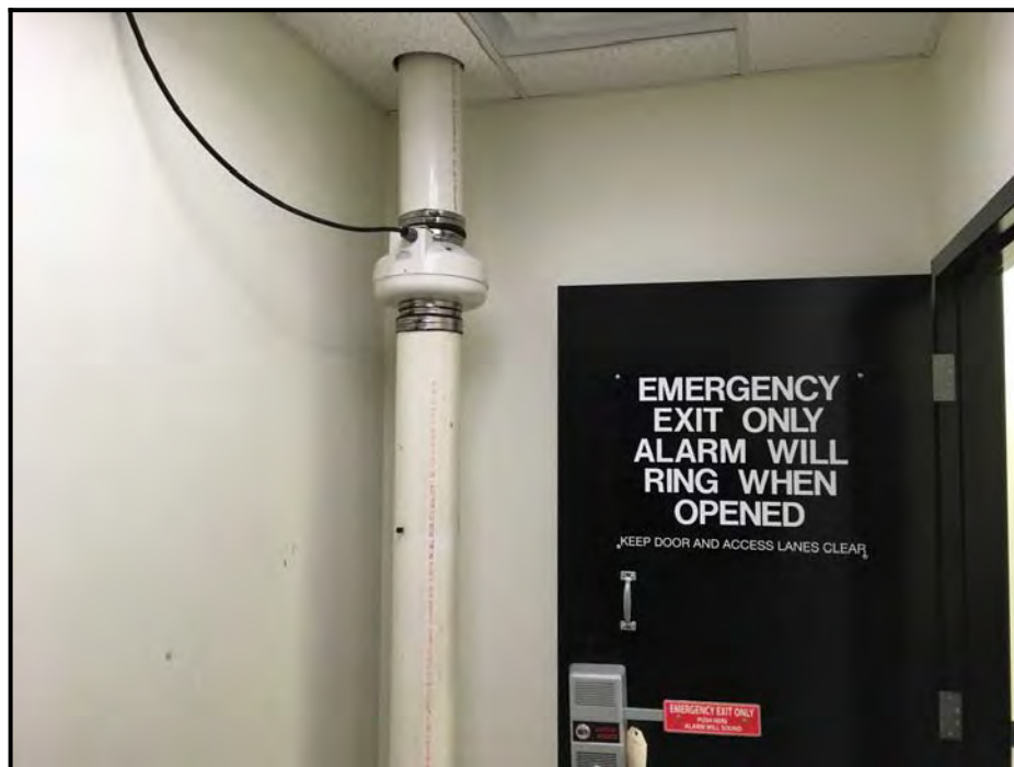
The west SSDS in a back room at Karma store.
