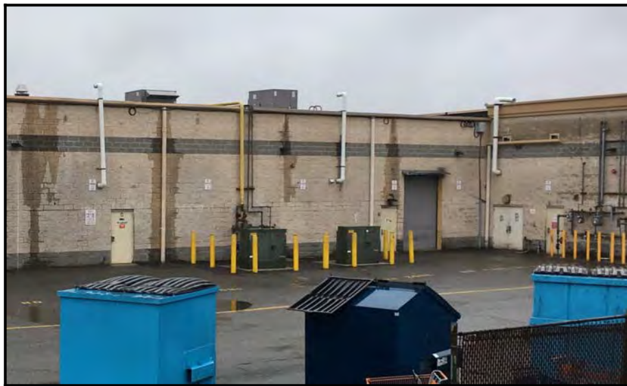
The white exhaust pipes for Karma (left and center) and the manifold pipe for the North Hallway (right). All SSDS exhaust points are located greater than 10 feet from any HVAC intake.
