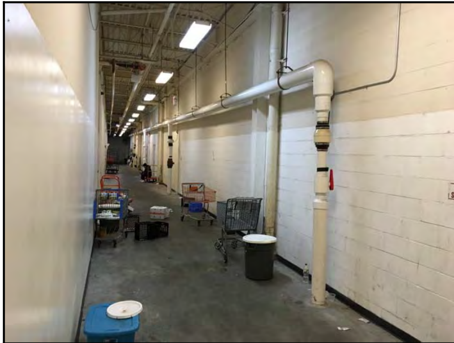
The North Hallway SSDS and its lateral manifold pipe.
