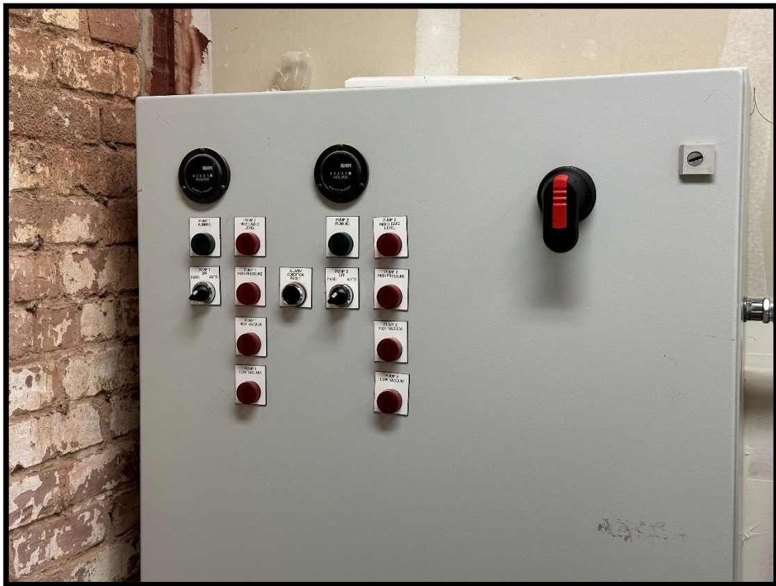
Photograph 3: Photo of active Factory SSDS Blower control panel.
