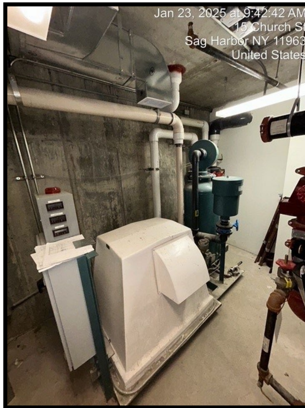
Photograph 19: Photo of garage SSDS Blower overall unit system equipped with inlet filter, knockout tank, monitoring point meters.
