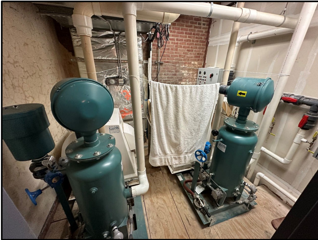
Photograph 5: View of two (2) SSDS Blower configurations with inlet filters, knock out tank, and control panel in view.
