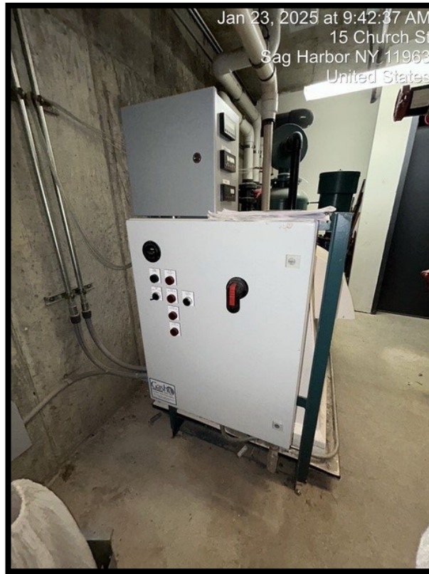
Photograph 11: View of garage SSDS Blower control panel and monitoring point meters in operation.
