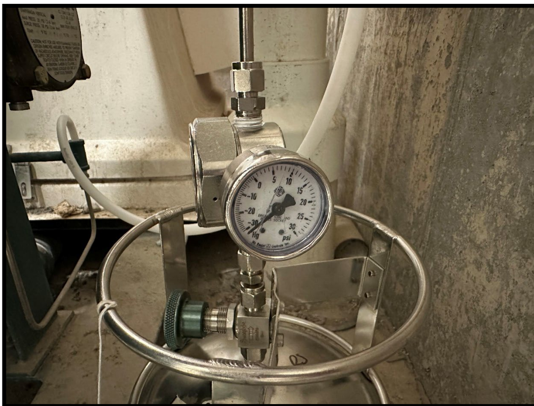
Photograph 10: Photo of effluent soil vapor sample pressure readings for Garage SSDS.
