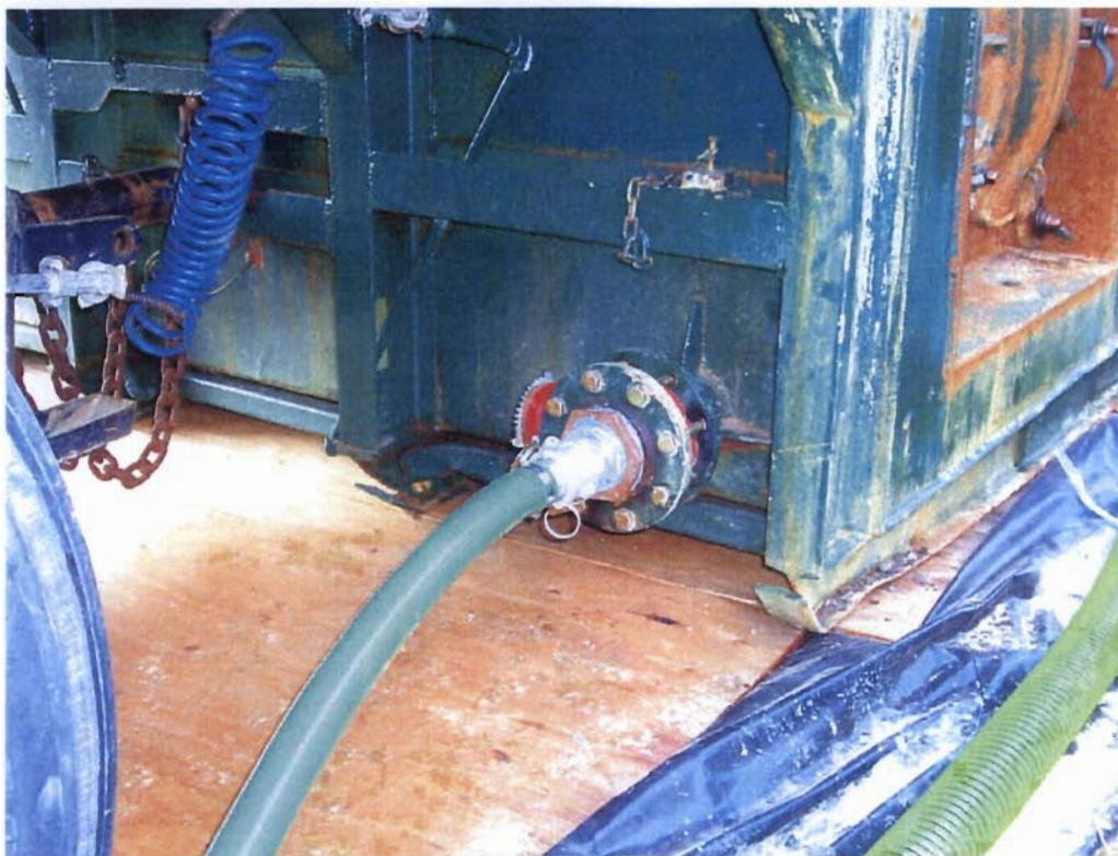
Photo #5: Connection pipe from batch mix tank to permanganate injection pumps.
