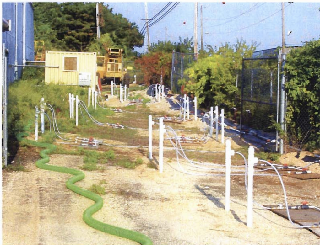
Photo #8: Permanganate injection wells.
