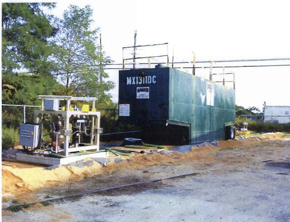
Photo #3: Potassium permanganate feeder mix unit (left) and permanganate batch mix tank (right).
