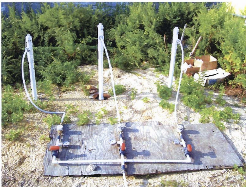
Photo #9: Manifold legs from header pipe to injection wells.
