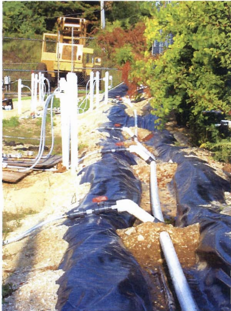
Photo #7: Header pipe (in lined berm) from permanganate injection pumps to injection well manifold legs.
