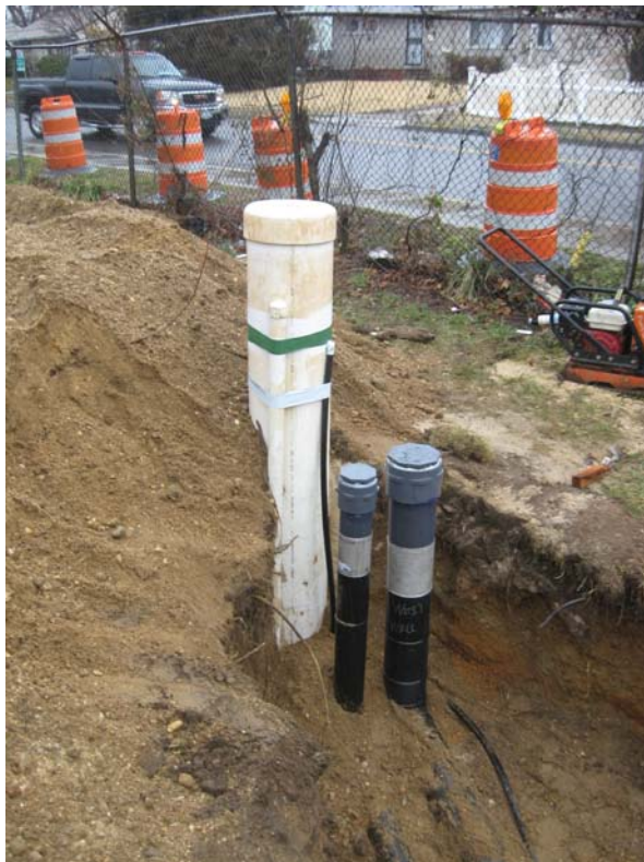
View of DDC-06 with 4-in. air supply and 6-in. air return lines. Note: Black condensate line attached to well.
