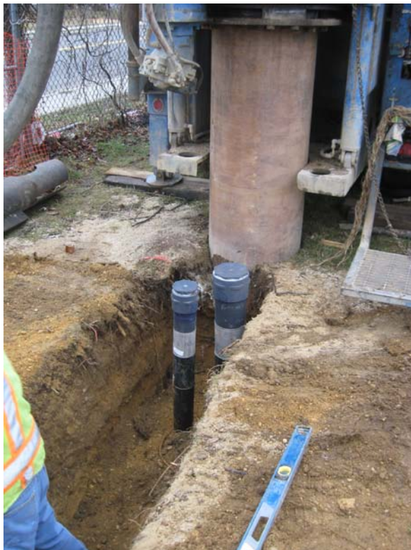
View of 4-in. and 6-in. air lines at DDC-05.
