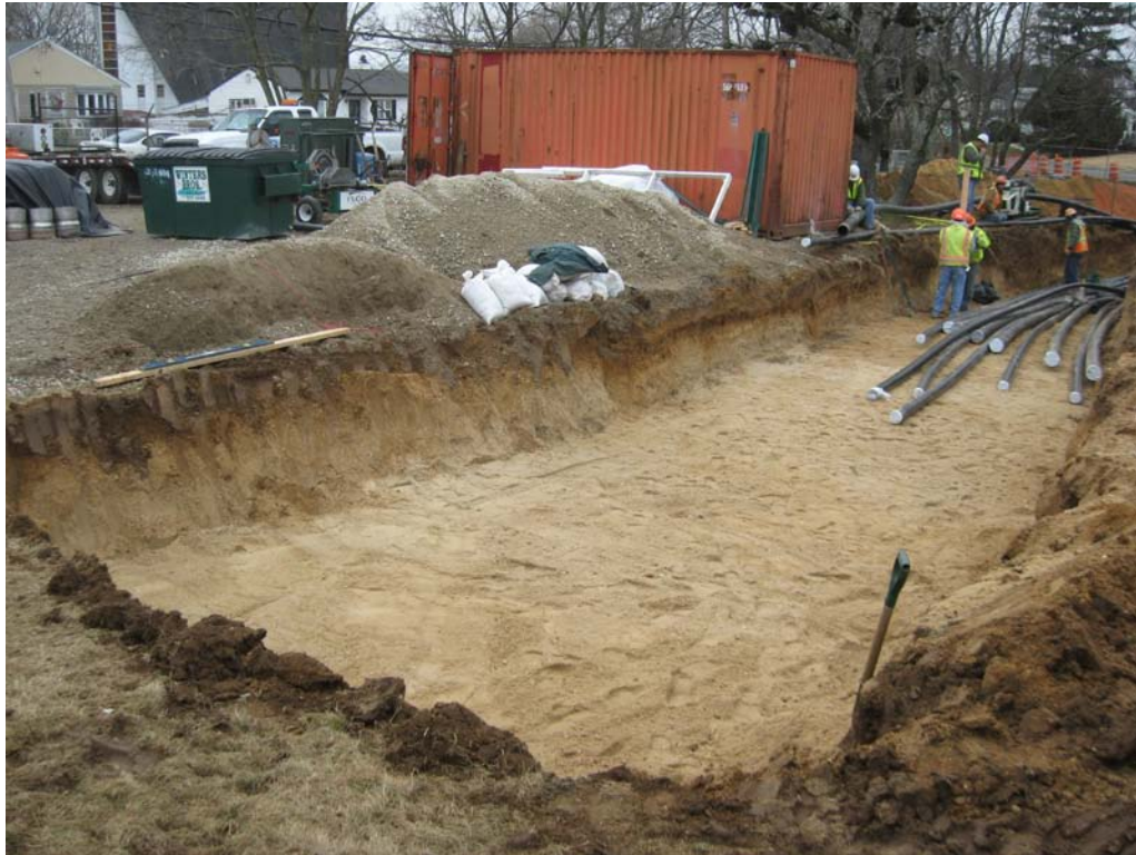
View of treatment system pad and trench line.
