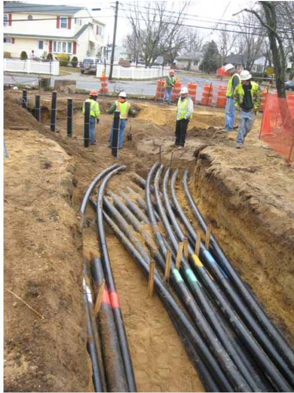
View of 4-in. and 6-in. lines merging together, looking west.
