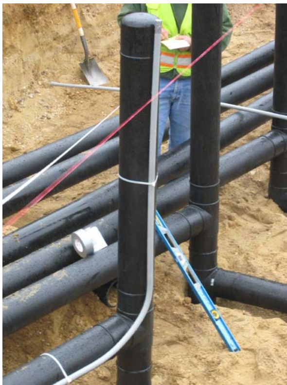
View of electrical conduit piping attached to sump.
