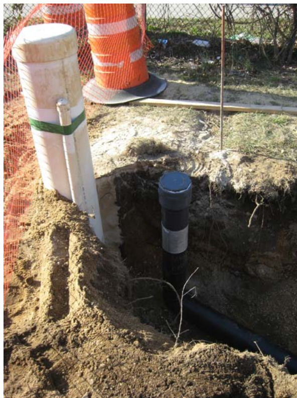
View of 90-degree 6-in. return line at DDC-06.
