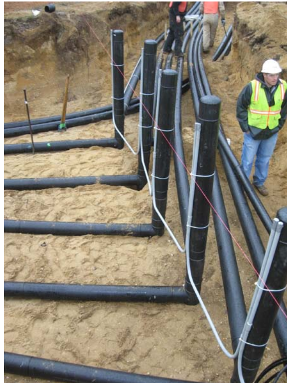
View of electrical conduit piping attached to sumps.
