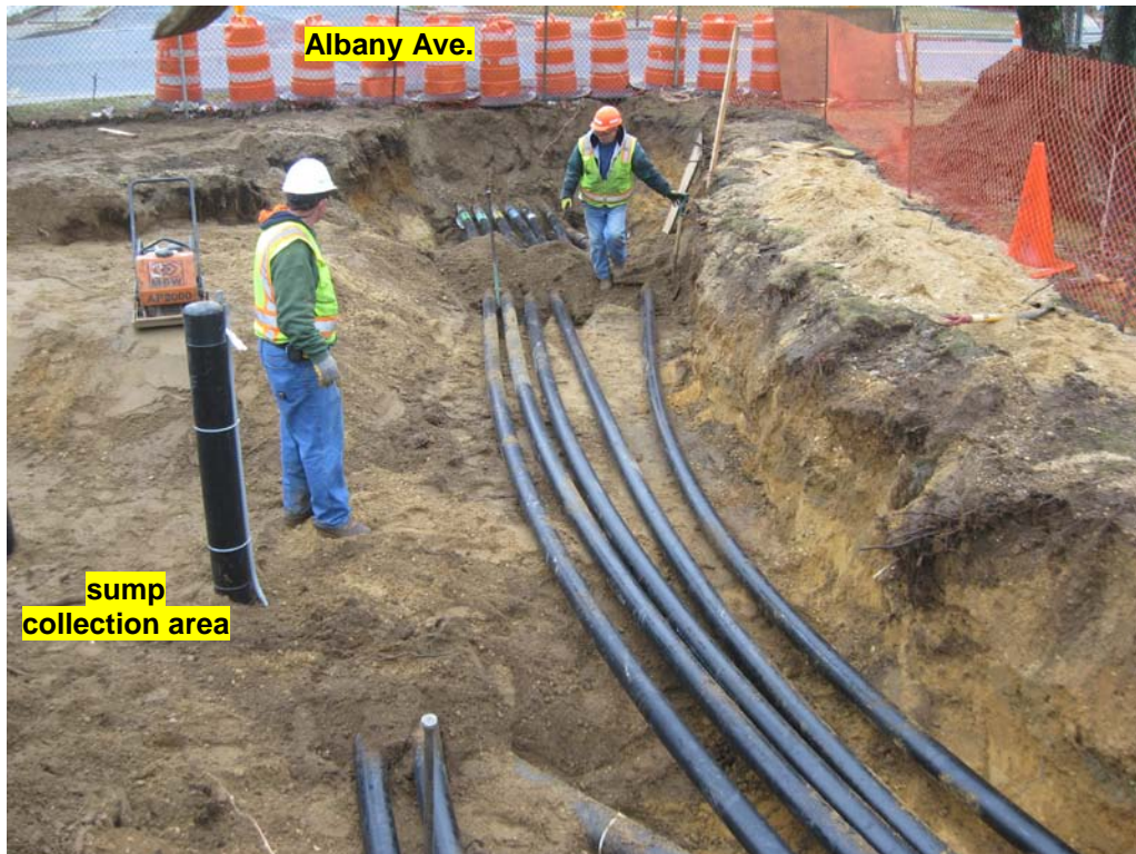
View of 4-in. lines bypassing sump collection area.
