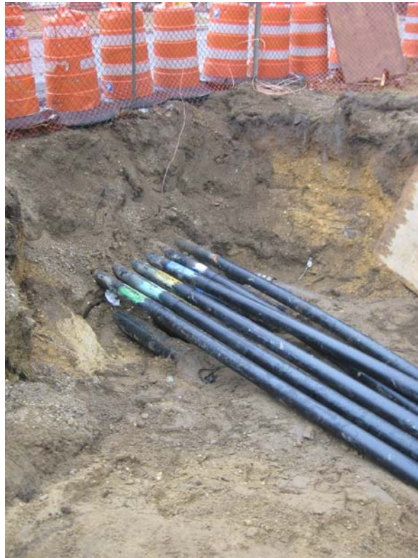
View of 4-in. air supply lines extending from Benjoe Dr.
