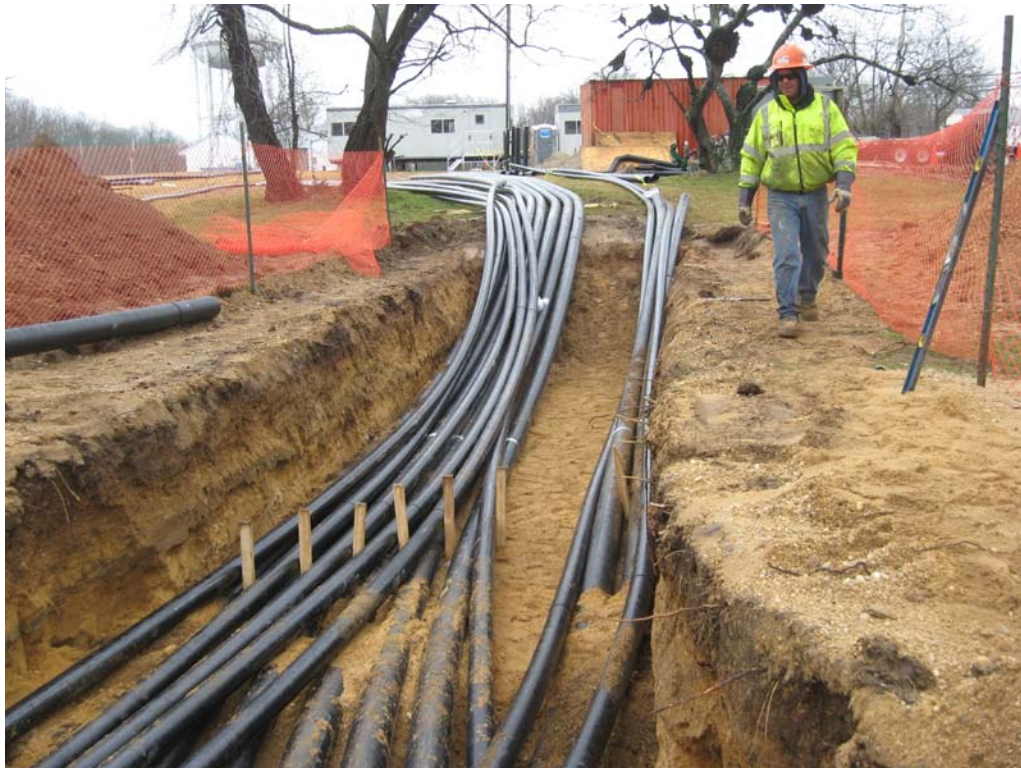
Air lines extending to the east towards treatment system pad.
