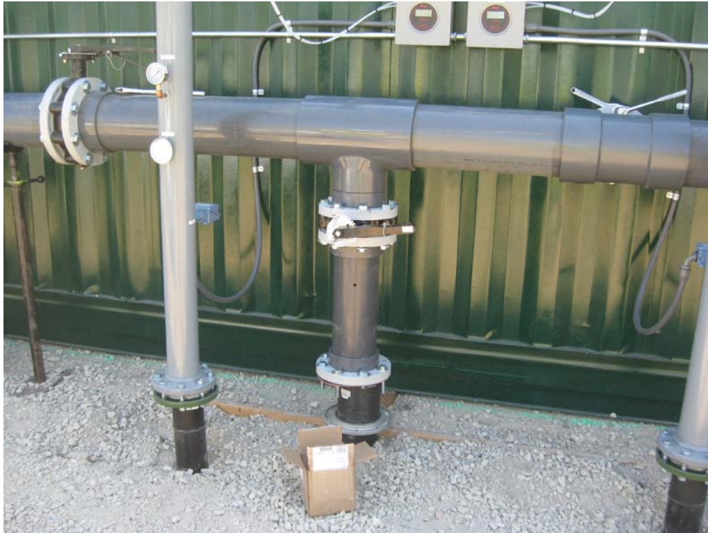
View of 6-in. air-return line connection to Treatment Trailer #1 manifold.
