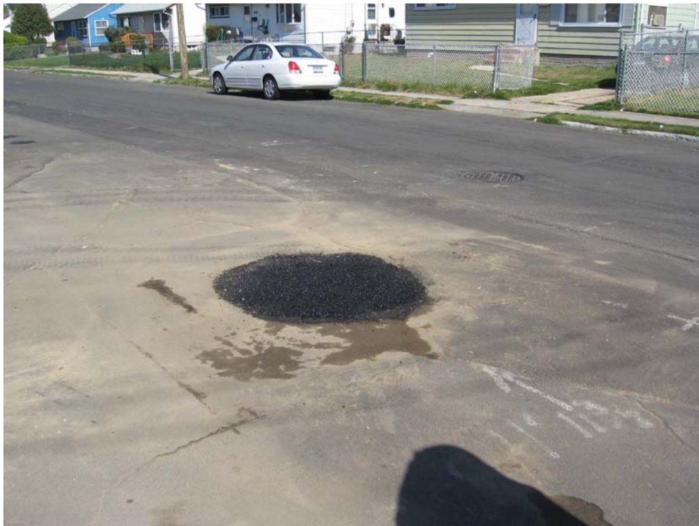
View of temporary asphalt patch at DDC-09, looking northeast.
