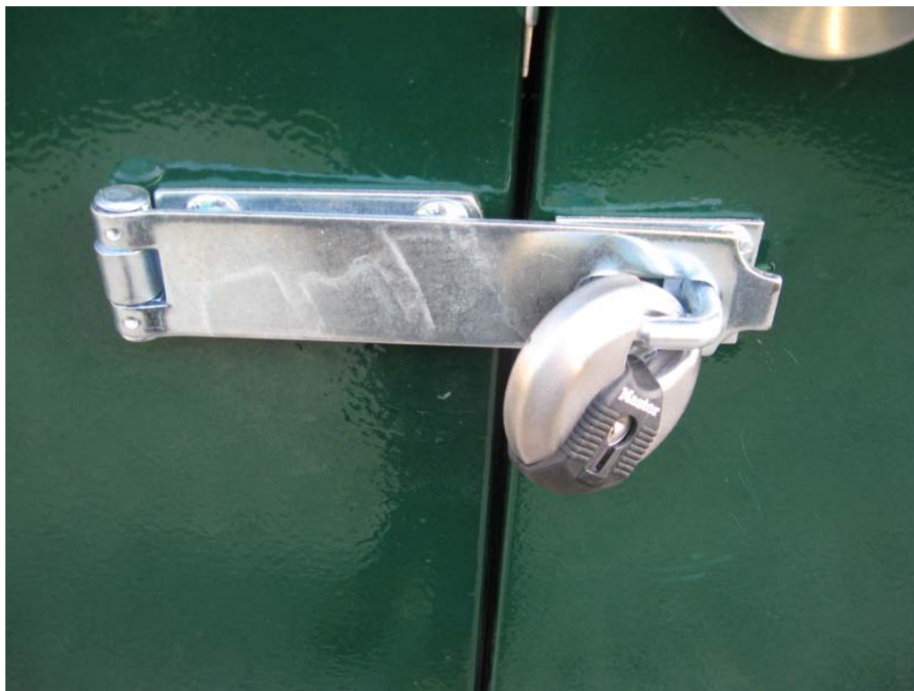
View of latch and lock installed on access door to Treatment Trailer #1.
