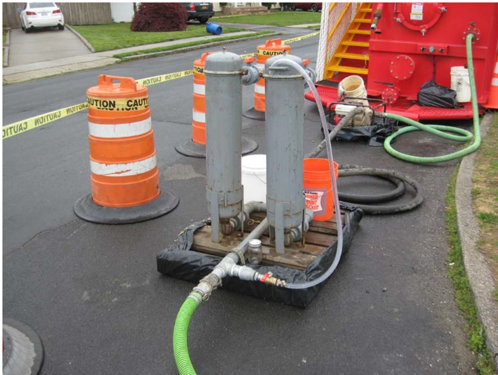
Two vessel filtration system mounted on secondary containment.
