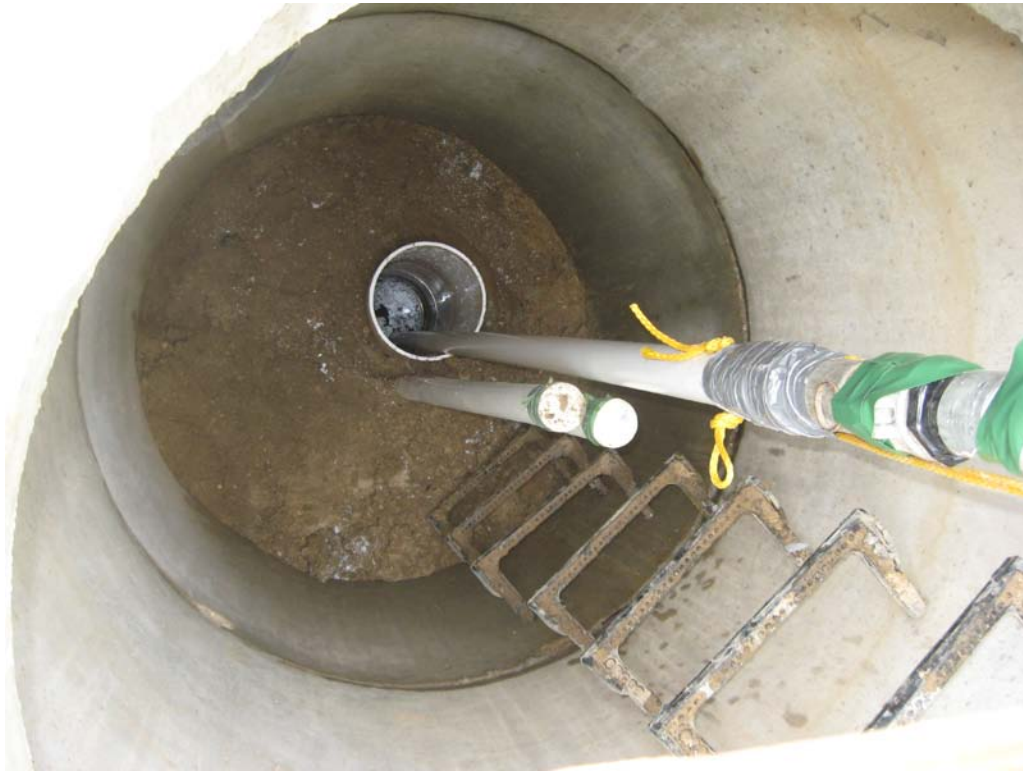
View of DDC-10 vault with centrifugal pump lowered into recirculation well.
